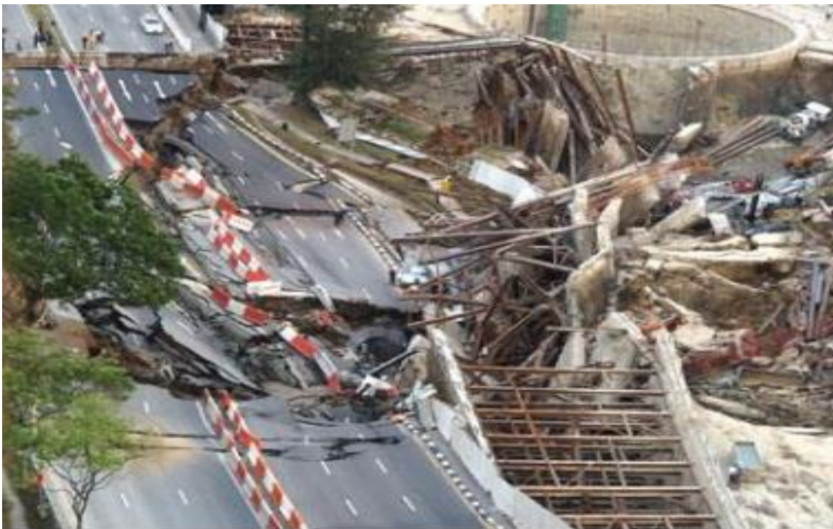
Figure 1: Singapore Nicoll Highway collapse adjacent to an excavation (Yuepeng Dong, 2014)
