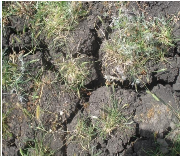
Surface cracks formed during drying of swelling clays, Feb, 2012
