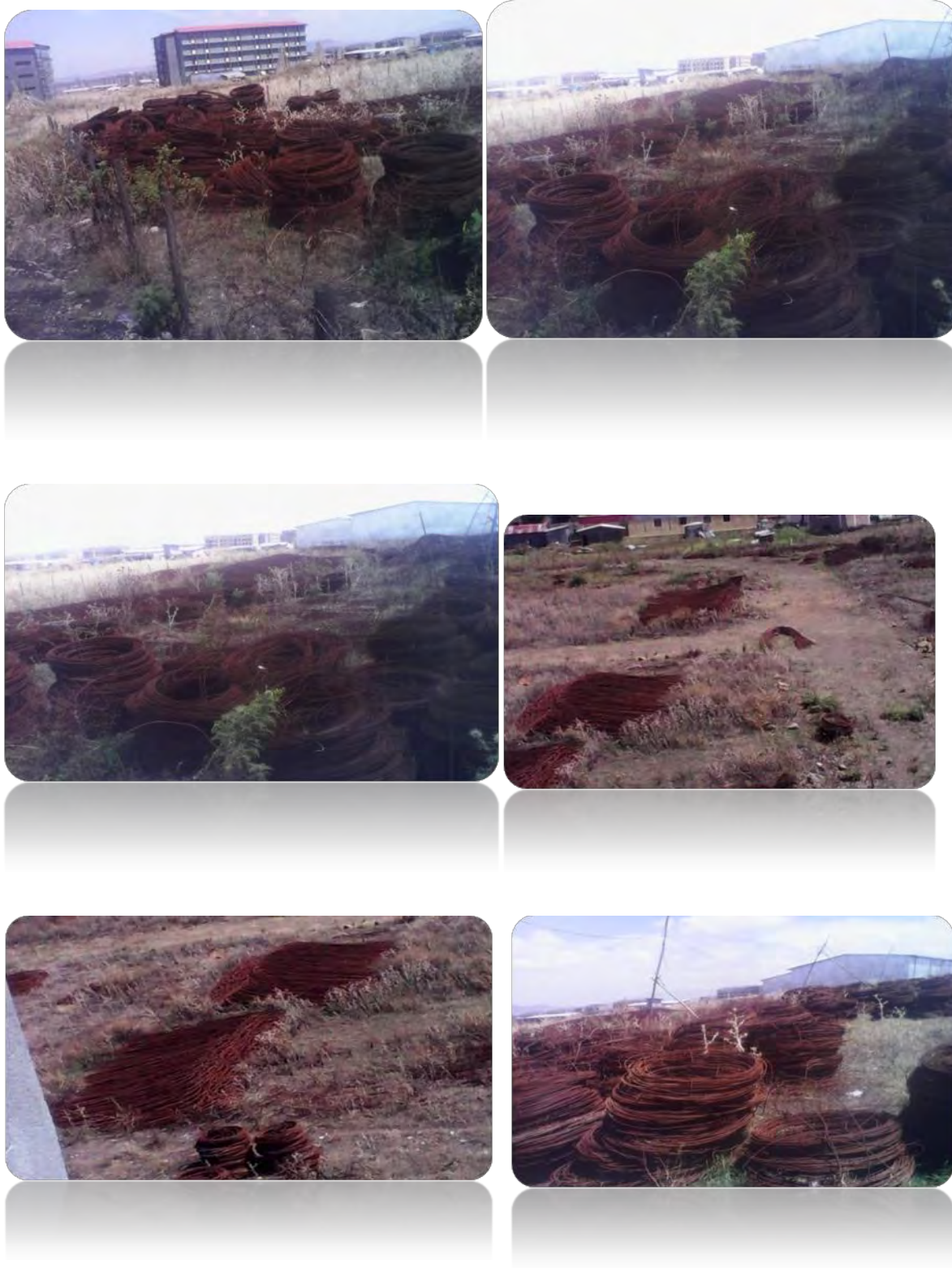
Figure:- 4.5 Poor handling of steel reinforcement bar on building construction site
