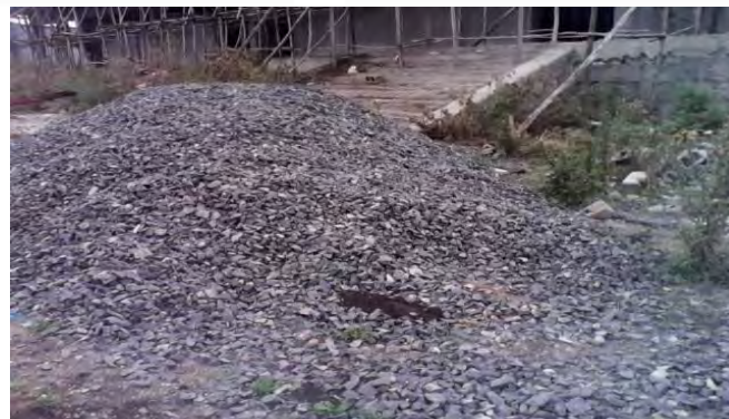
Figure: - 4.7 Poor handling of Coarse aggregate onsite
