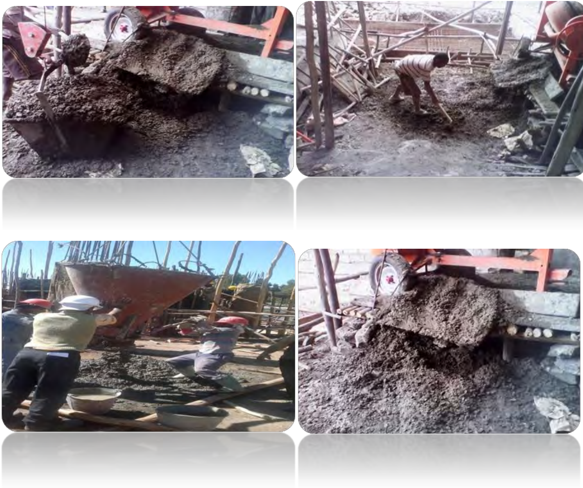
Figure: - 4.9 Wastage of concrete due to Poor transport
