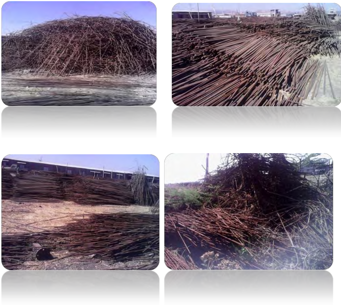
Figure:- 4.4 wastage of steel reinforcement bar due to Non-optimized cutting of bars and design change
