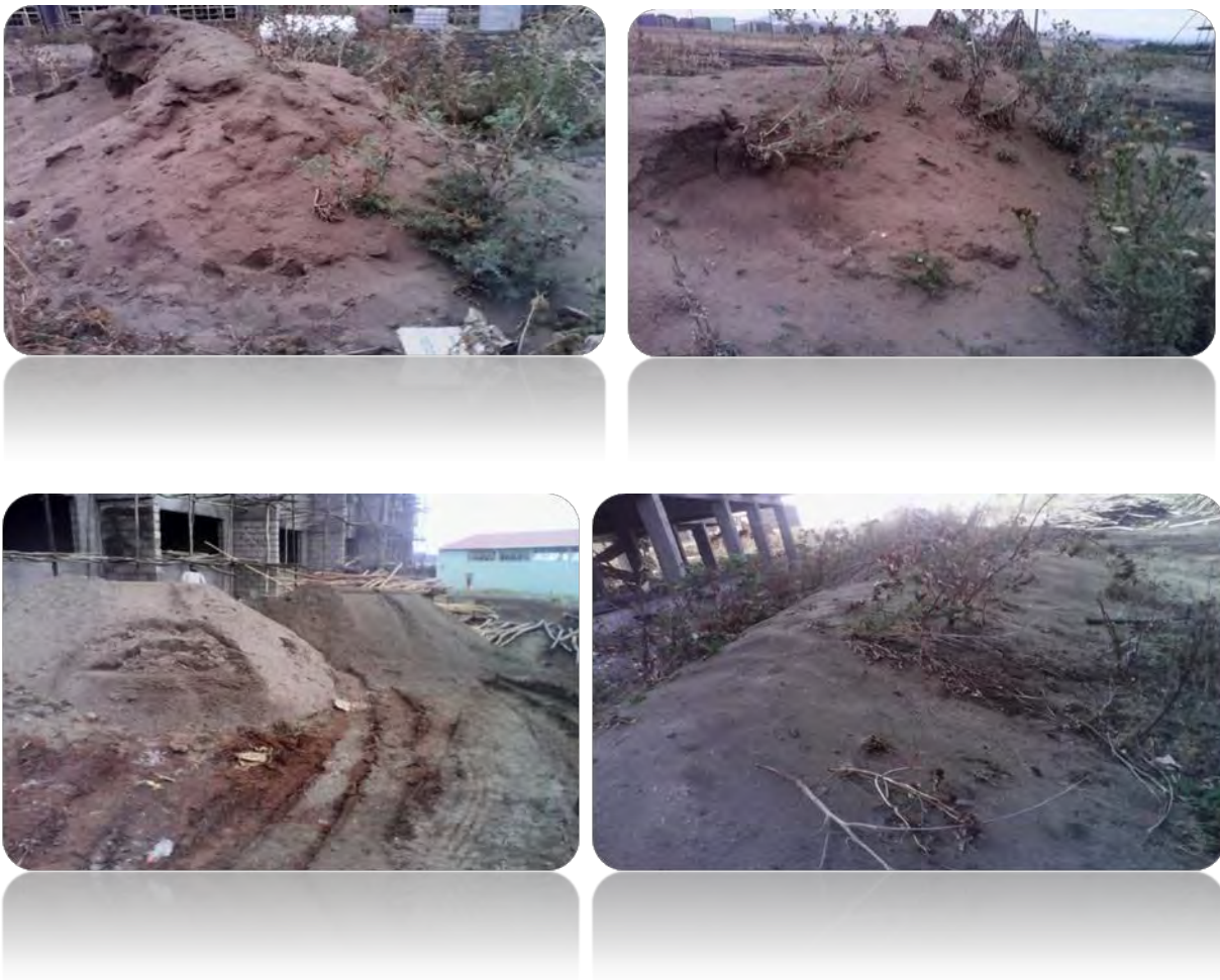
Figure: - 4.6 Poor handling of sand onsite
