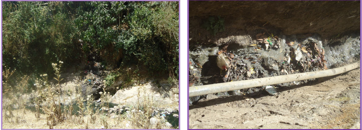
Pic 4.13 open ditches and river bed filled with liquid and solid wastes, producing repulsive odor
