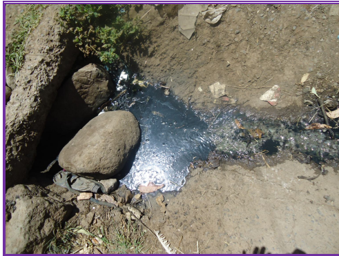
Pic 4.5 open ditches clogged by wastes
