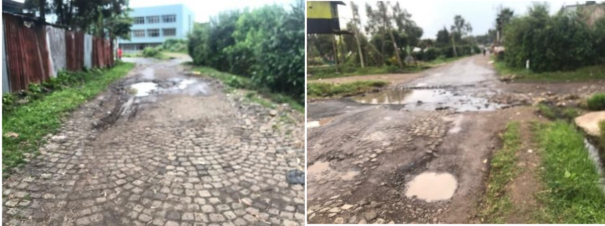
Figure 6: The Study site in Akaki Kality Sub city with cobblestone road features, damaged surface areas (right side) and adjacent road to the site contributing runoff (left side).(Source: photograph taken by the author on August 2019)
