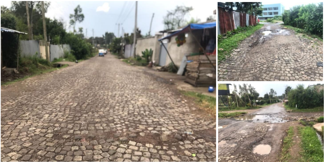
Figure 39: The Study site in Akaki Kality Sub-city with cobblestone road features, damaged surface areas (bottom right), and (Top right) adjacent road surface to the site. (Source: photograph taken by the author on August 2019)
