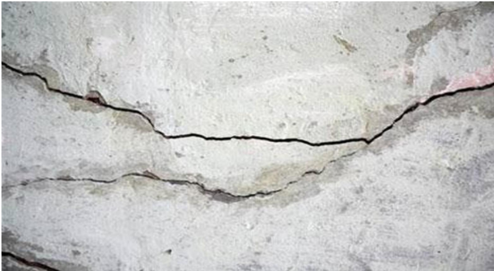
Figure 2.3: Cracking of concrete (Eng. Sdeiq Jalal Abdullah, 2013)
