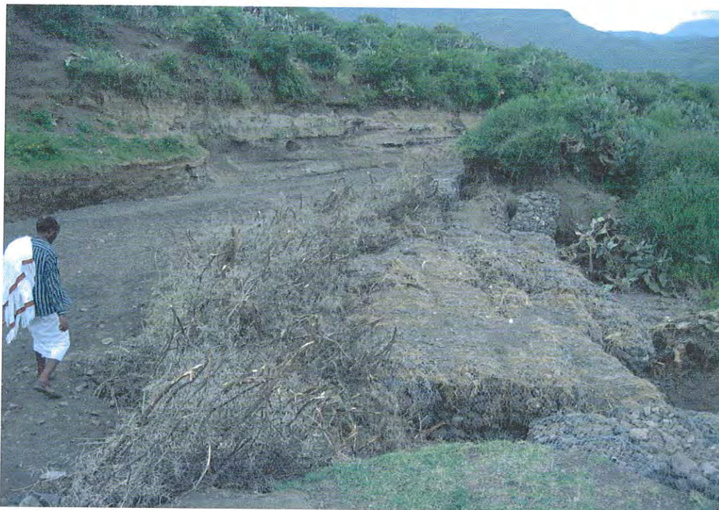
Plate 5.3: Damaged primary canal at Boboteya spate irrigation system
