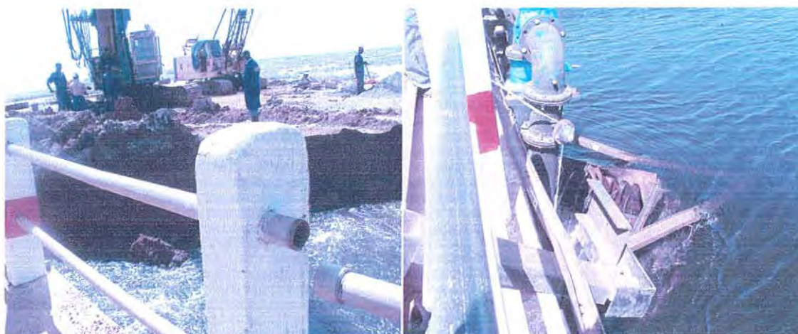
Figure 7.1: Road works at the main NWSC water pumping site in Aoja Swamp Soroti
