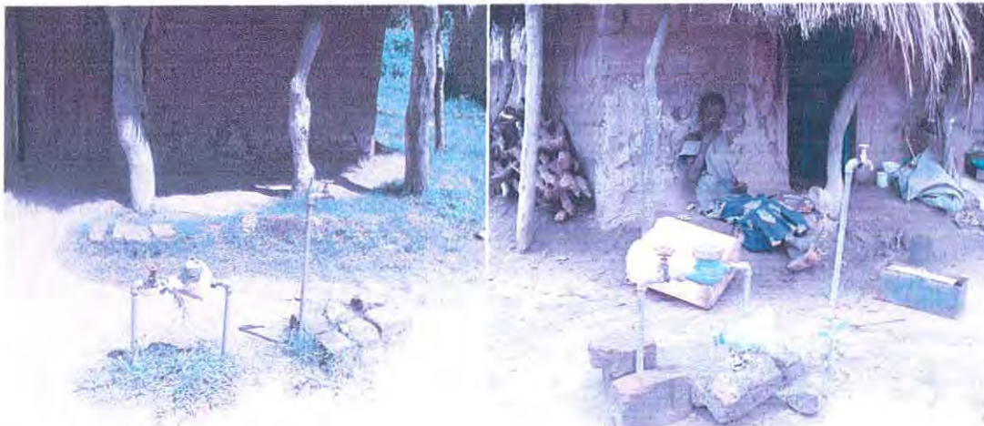
Figure 6.1: Water connections to the low-income households in ATC, Central ward
