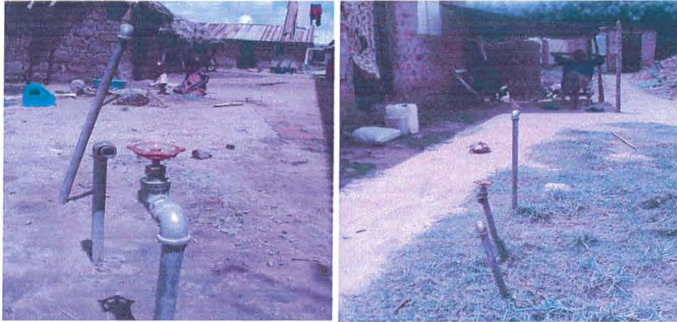
Figure 5.6: Some of the households’ yard piped water disconnected in ATC
