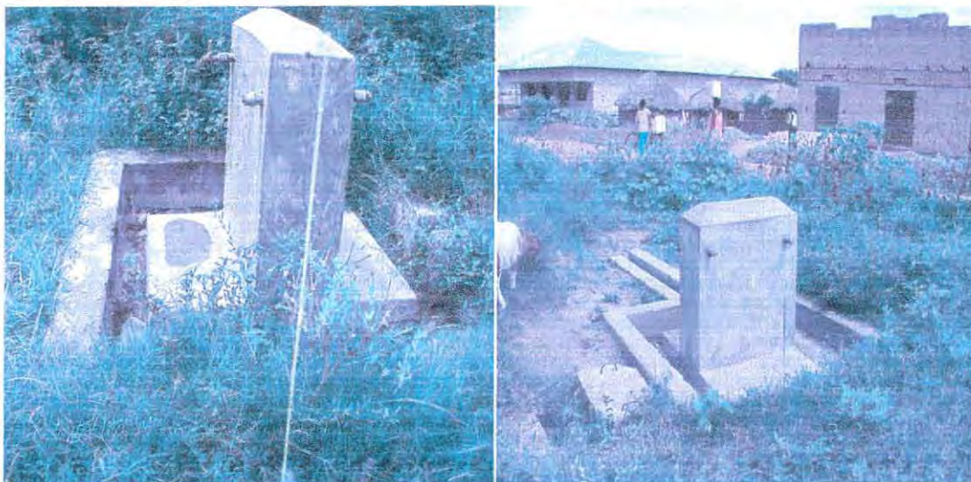
Figure 5.9: Examples of non-functional public stand pipes in Central Ward ATC.
