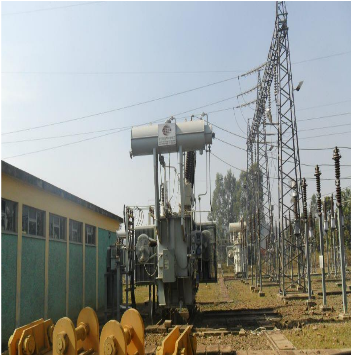
FIGURE 3.2: Jimma old substation
