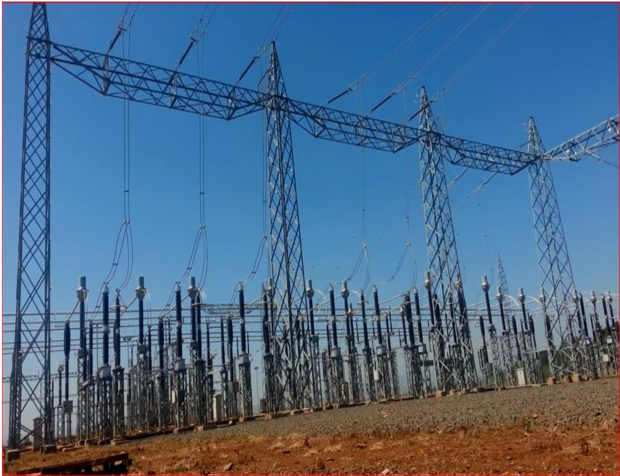
FIGURE 3.5: JIMMA NEW SUBSTATION
