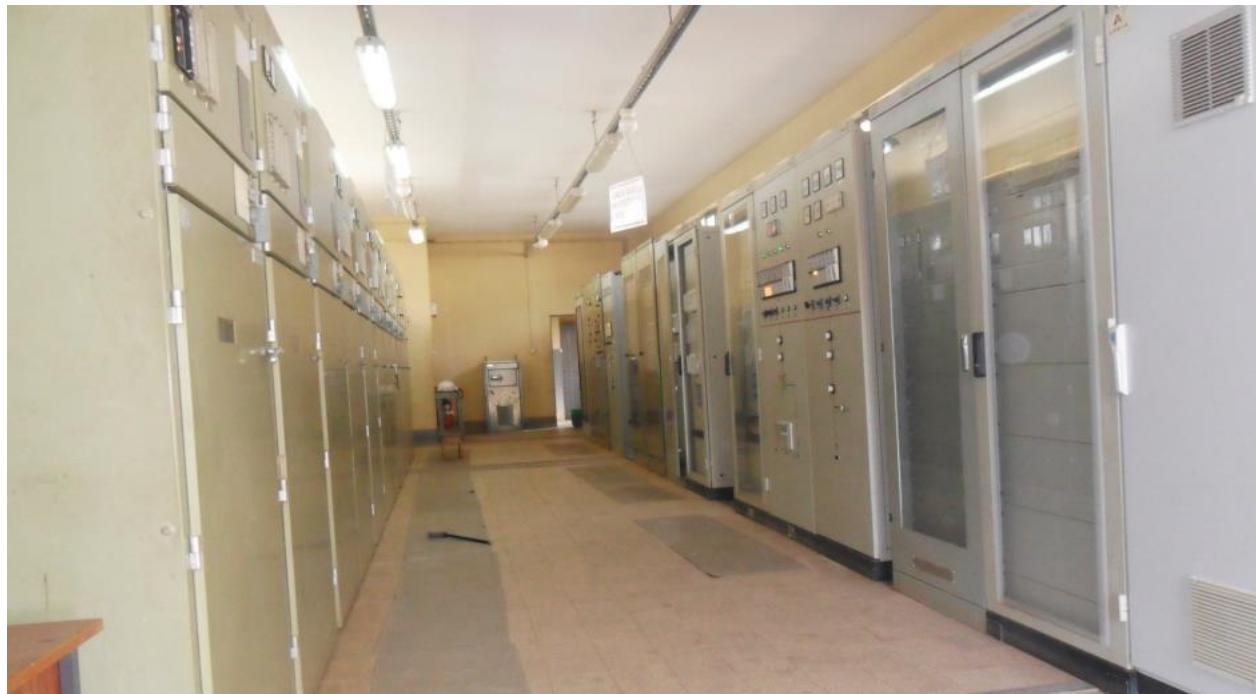
FIGURE 3.4: JIMMA OLD SUBSTATION CONTROL ROOM
