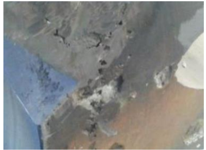
(f) Surface crack
