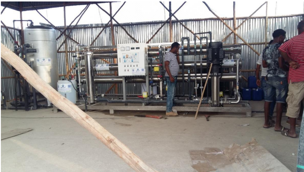
Water Treatment Plant ~ Cap. 1200 lit/hr
