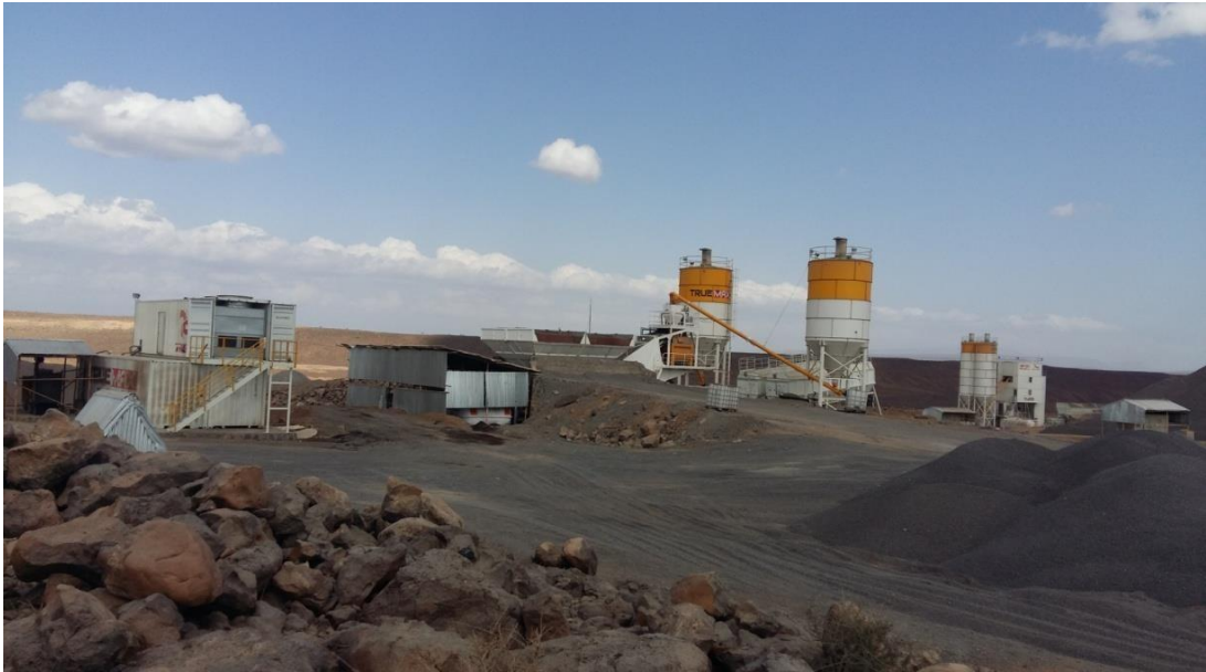
Batching Plant ~ Av. 60 M3/hr
