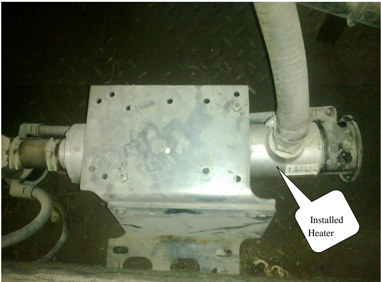
Figure 4.5: Installed Electric Water Heater (Source: Picture taken on site)
