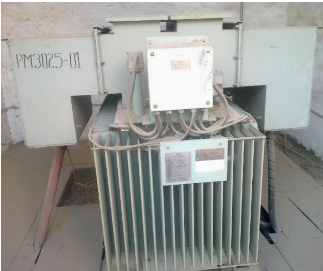
Figure 3.4: Step up transformer (Source: Picture taken on site)
