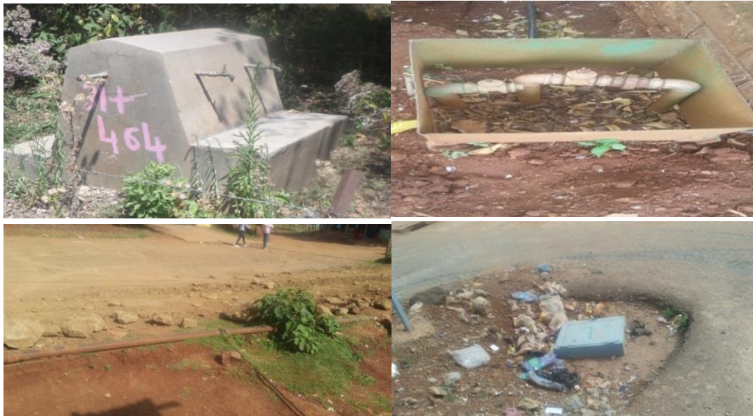
Figure 8: Photo of existing water point, junction and pipe line in the town
