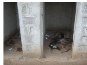
PPS-4 (Common latrine)
