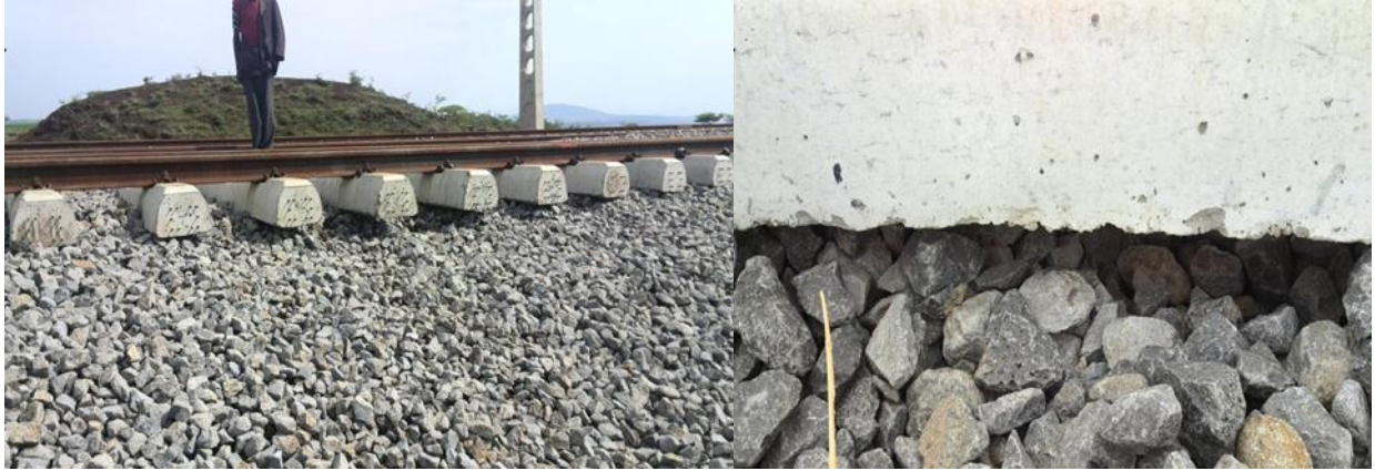
Unfilled ballast under the sleeper along Aama - Awash section [23]
