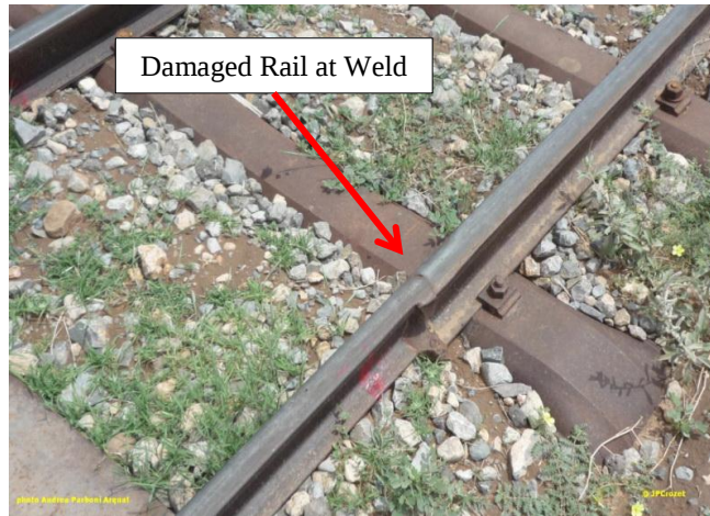
Damaged Rail at Weld, Ethio-Djibouti Railway Line 1964 [22]
