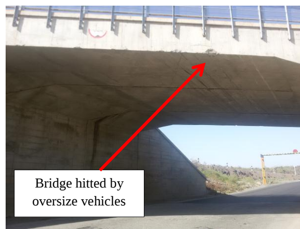
Bridge around Olenchity repeatedly hitted by oversize vehicles, ERC
