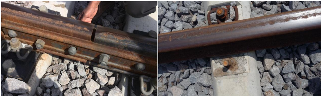
Loose and missing bolts around Metehara and Olenchiti [23]
