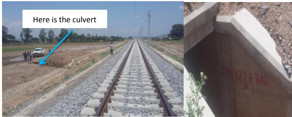
Poor Culvert design at location 137 DK, around Olenchiti sleeper factory [23]
