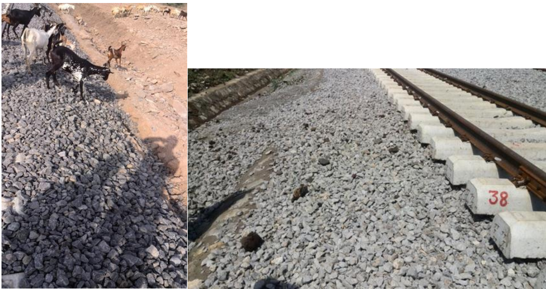
Lack of uniform width of ballast section; too narrow and too wide respectively Adama-Awash [23]
