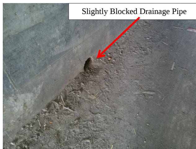
Slightly Blocked Drainage Pipe on bridge around Alemgena, ERC
