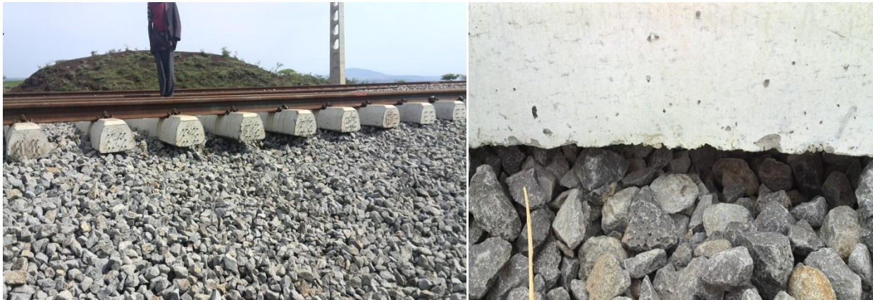
Unfilled ballast under the sleeper along Adama-Awash Section [23]
