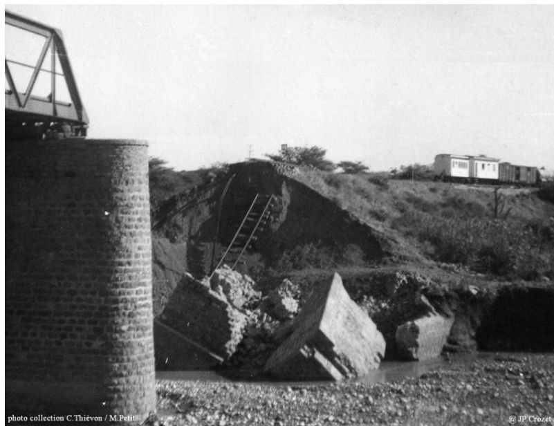
Figure 2-16: Bridge Failure due to scoured abutment 1955 [22]
