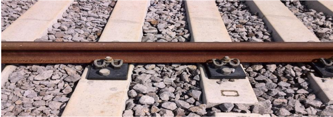
Corrosion of rail along Aama - Awash section [23]
