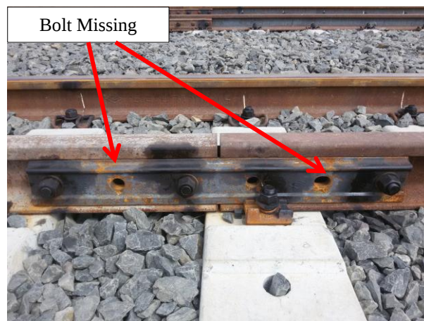
Bolt Missing, Around Alemgena ERC
