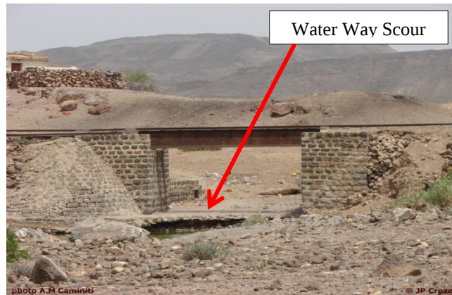
Water Way Scour bridge located around Awash 2008, Ethio-Djibouti Railway Line [22]
