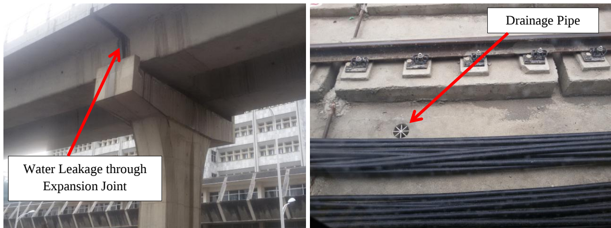
Water Leakage through Expansion Joint and Drainage Pipe in Good Condition, AALRT around Legehar
