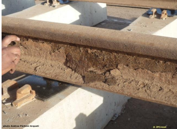
Corrosion of Rail, Ethio-Djibouti Railway Line [22]
