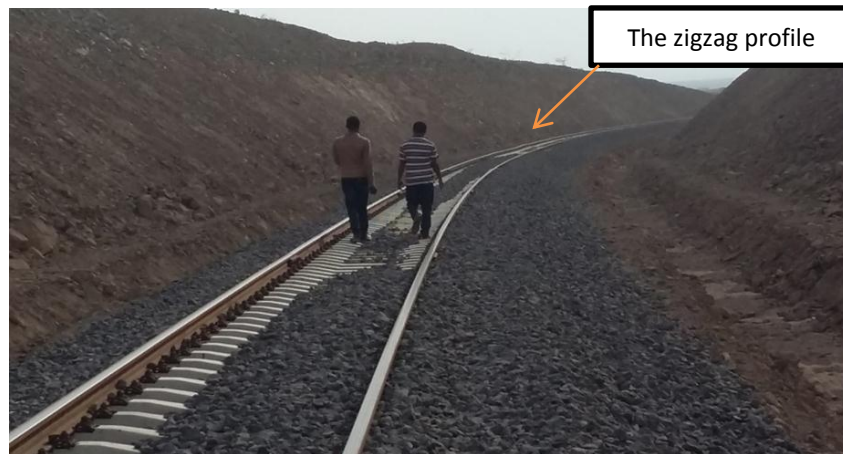
Rail at curve section, showing longitudinal irregularity and lack of guard rail along Aama - Awash section. [23]
