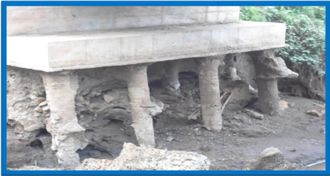
Photo1-2: Exposed Pile and Pile Cap due to Scour (Source: ERA, BMS-October 2012)
