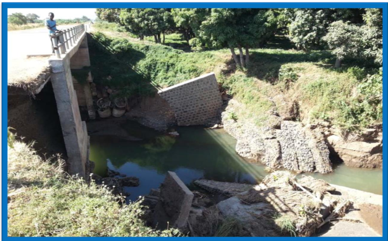
Photo1-8: Failed Right Bank Protection Work (Source: ERA-BMS, October 2012)
