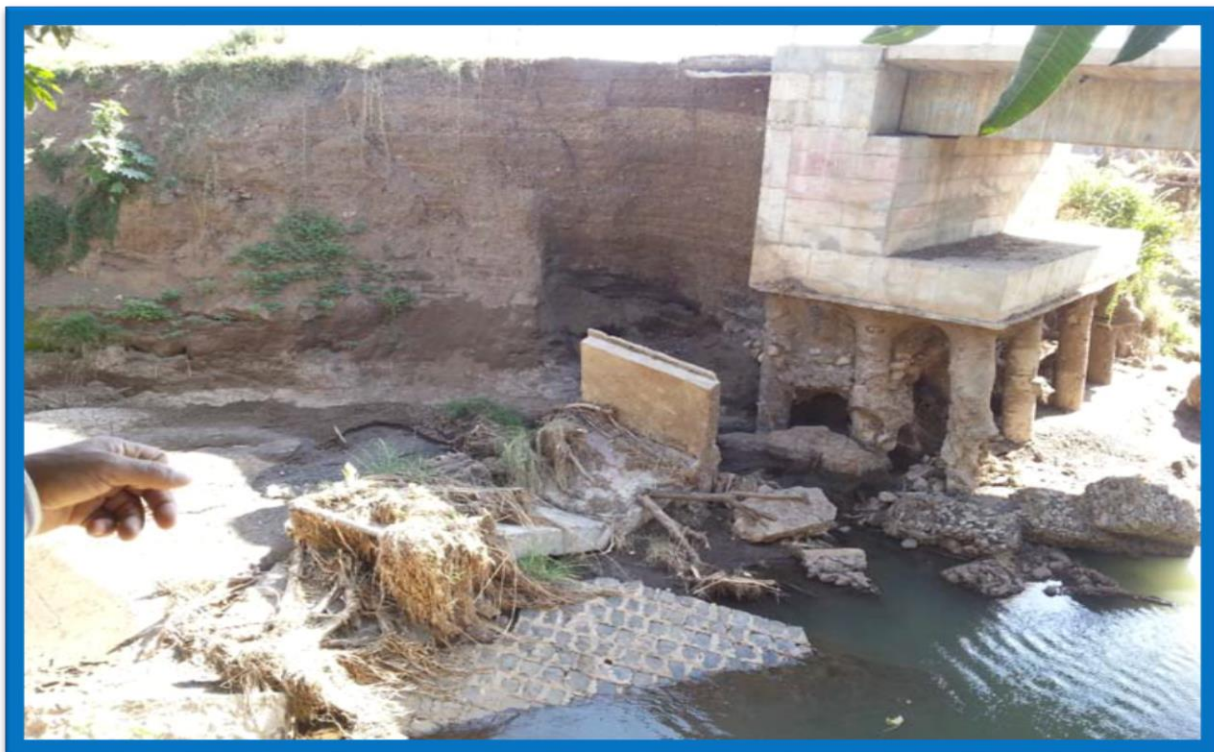
Photo1-6: Damaged Left Bank (Source: ERA-BMS, October 2012)
