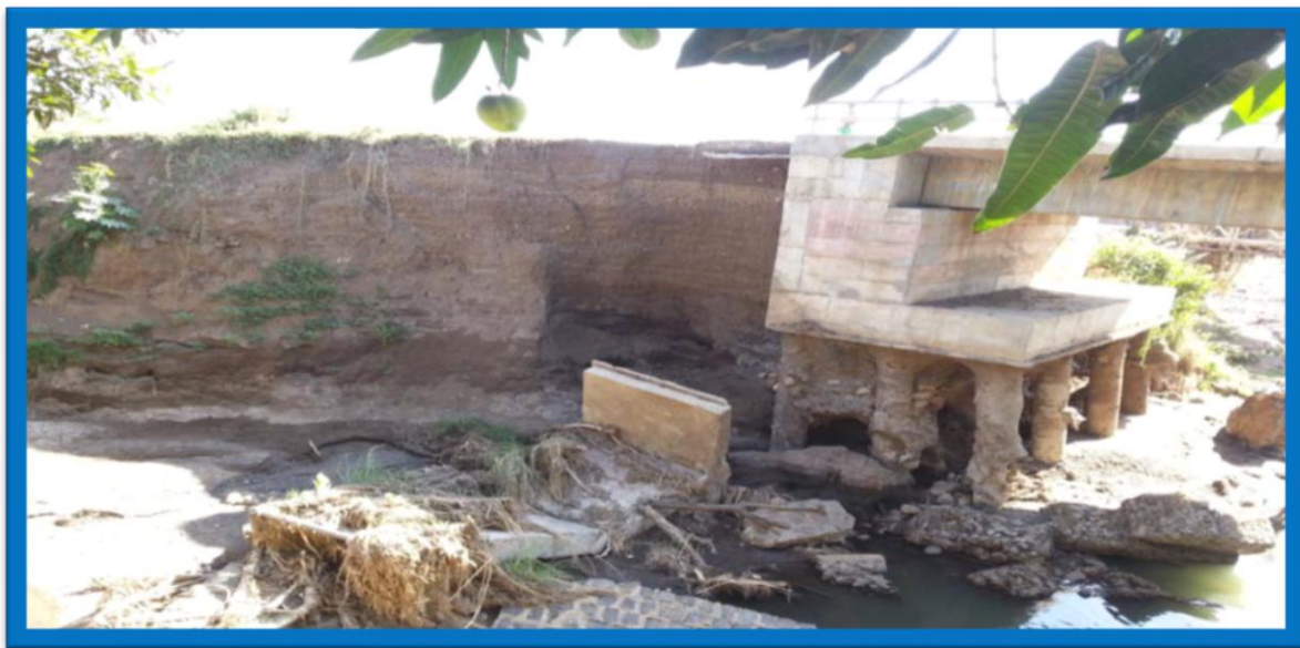
Photo1-3: Eroded Embankment on the Left Side of River Bank on Arbaminch Side (Source: ERA-BMS, October-2012)
