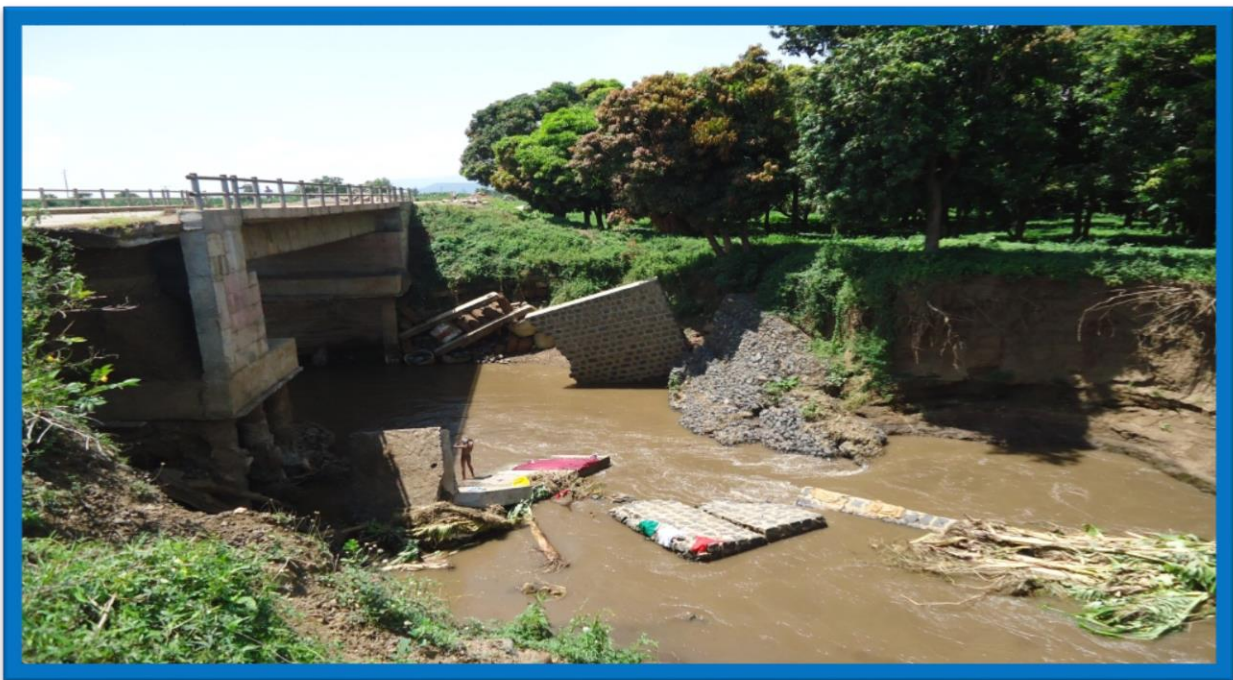
Photo1-4: Collapsed Protection work at the upstream Inlet Upstream
