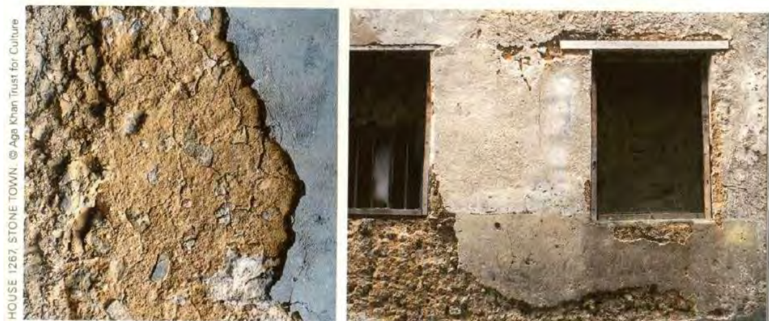
Figure 3-26 Identification of cement as an inappropriate restoration material, from Battle, Melin, and Forsman 2007
