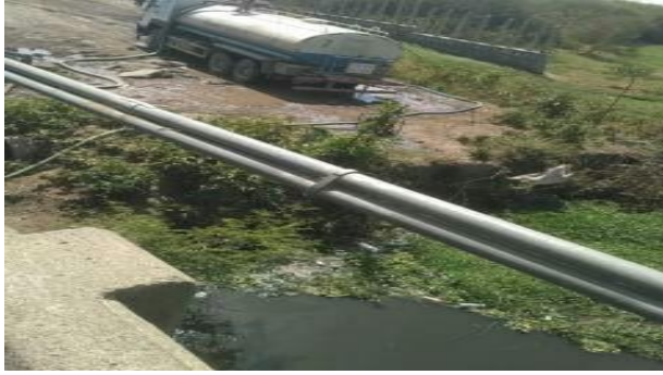
Figure 9. Up taking of water from the river for road construction purposes. [Photo courtesy by Hiwot Fiseha, 28/06/ 2010].
