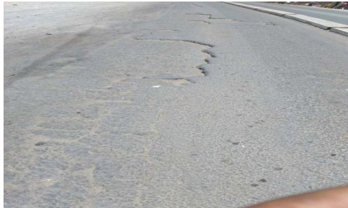
Photo 11 Poor Maintenance of road Outlet to Wonji Shewa
