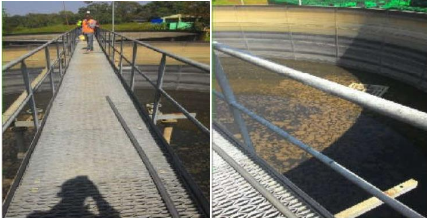
Figure 8: Bedele Brewery's Sedimentation Tank
