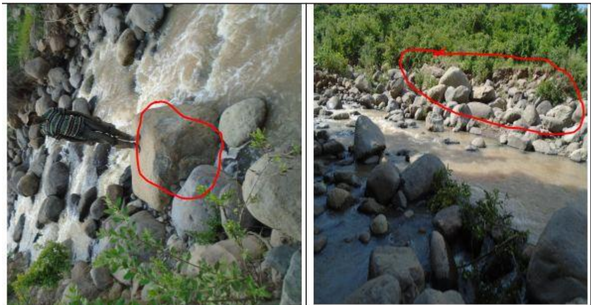
(a) Shows bolder of rocks at the left bank of the proposed site of diversion weir of Rufael SHP and (b) shows fine to boulder size transported material at the right bank of the proposed diversion weir site
