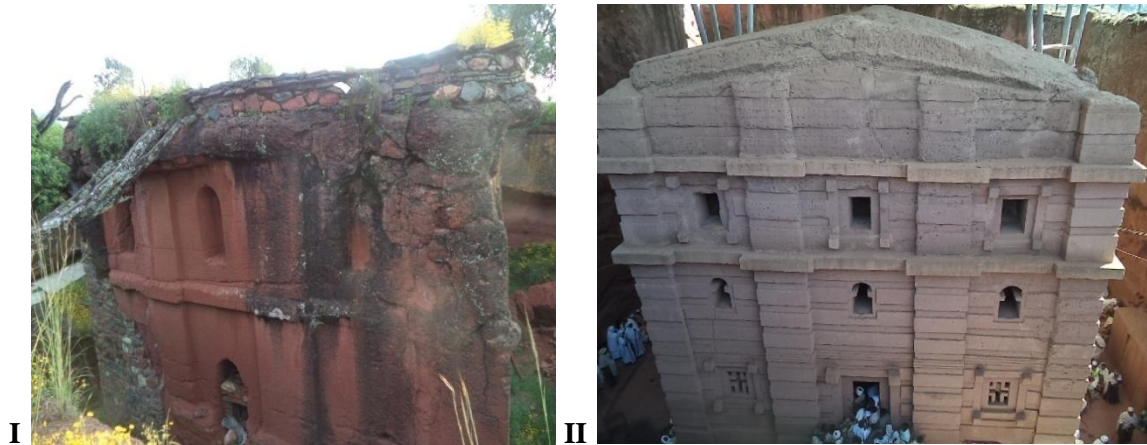
Fig.4.1 (I) the horizontal layers and buttresses on the eastern facade of Nazugn Maryam; fig. 4.1 (II) western facade of Bêtä Amanuel
