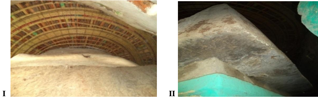
Fig. 3.11(I) the newly framed roof; fig.3.11(II) the edge of the main rock (the blue colored below the edge is the horizontal layer)
