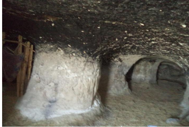
Fig. 3.28 poorly carved columns
