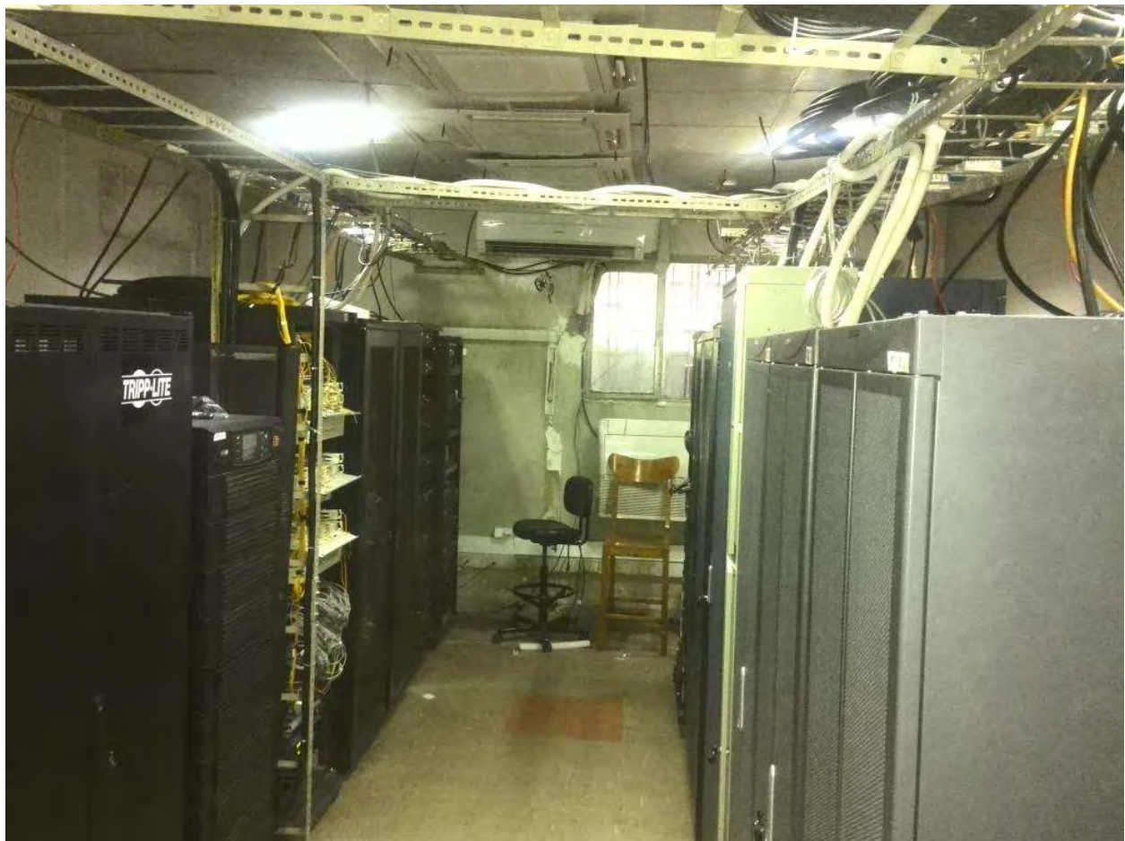
Figure 3-3 AAU Main Data Center
