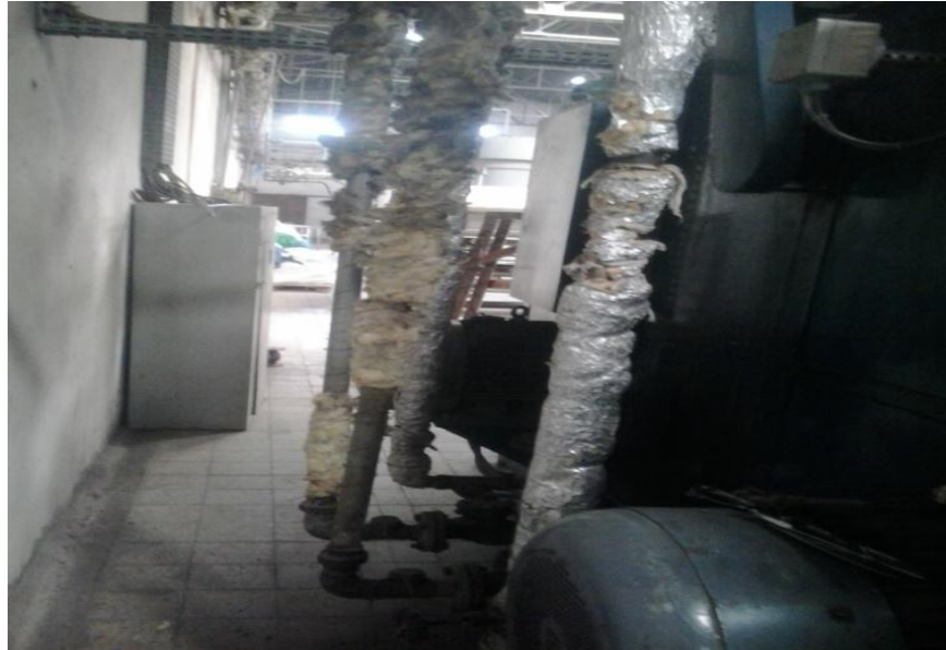
Figure 20 poorly insulated pipe
