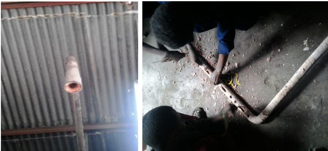
Figure 22 blocked water pipe and filter due to use of untreated water
