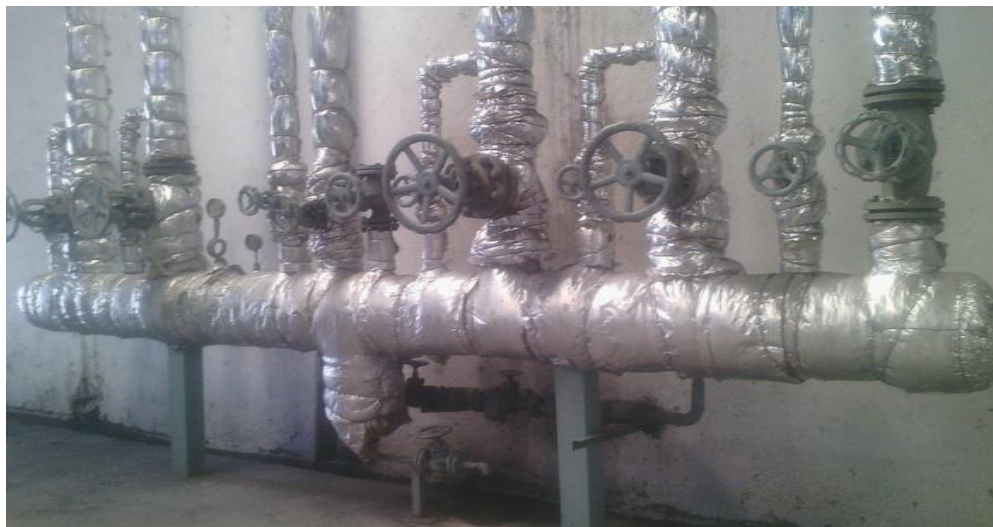
Figure 19 properly insulated pipe
