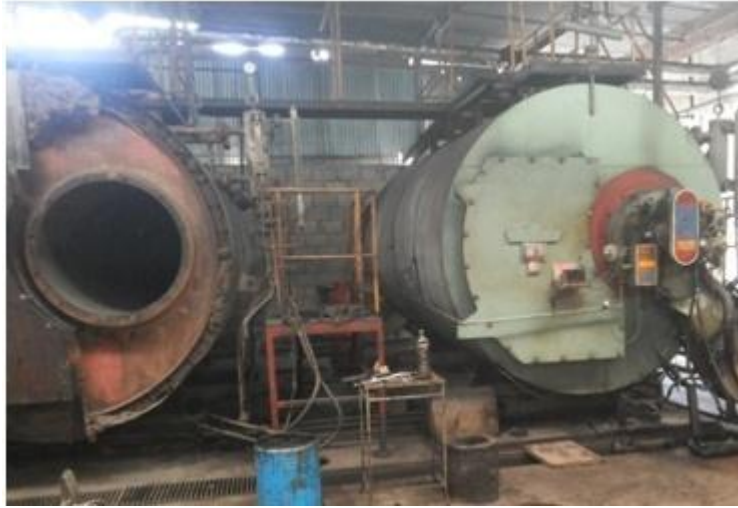
Figure 21 Burnt boiler due to use of untreated water
