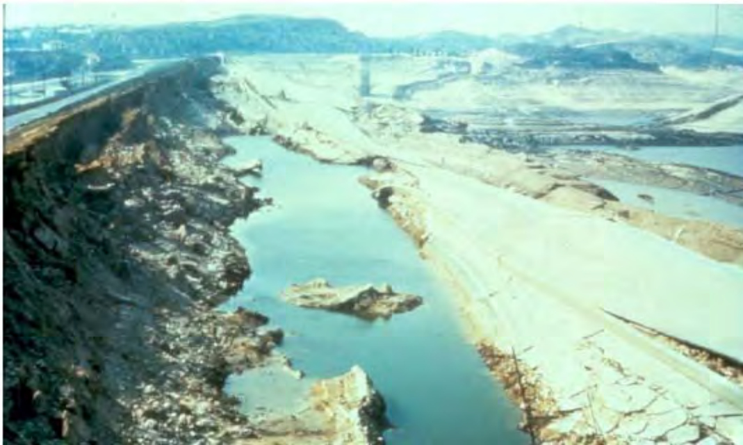
Figure 11: Liquefied lower Fernando dam upstream face
