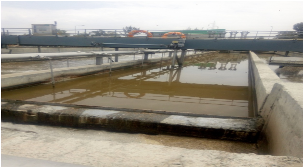
Figure 4-: photo of Kaliti WWTP taken during field observation, in 2019
