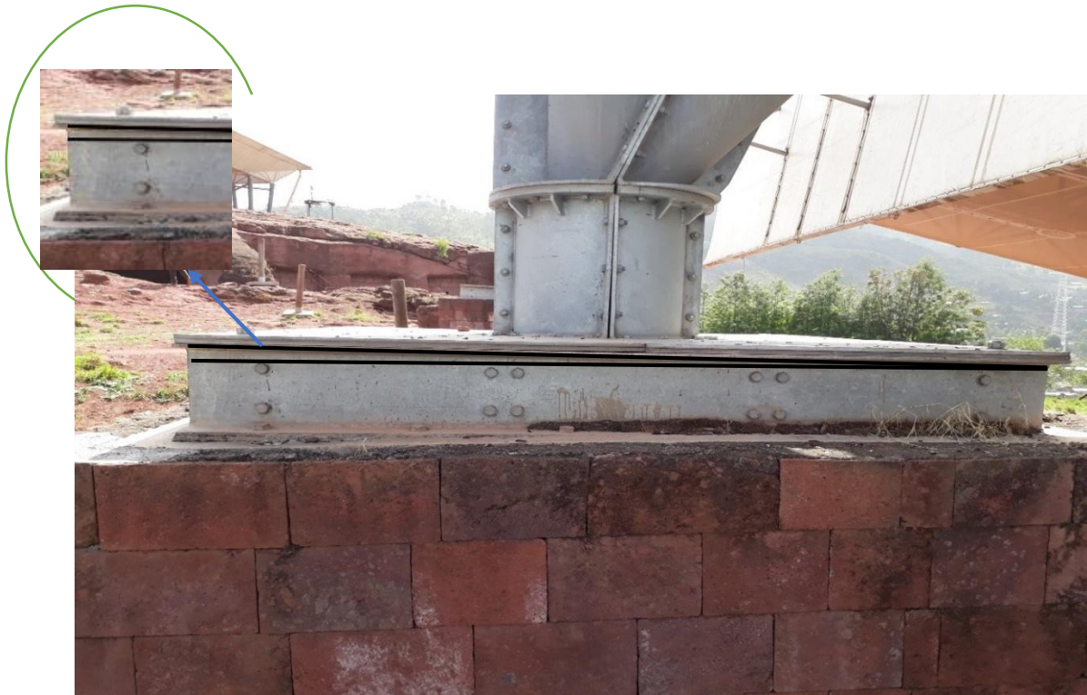
Figure 3.1.1-6 Column-C3 and C4 (There are no openings occurred between the plates but slight over turning of the base plates from the place where they bolted are witnessed in this two columns).
