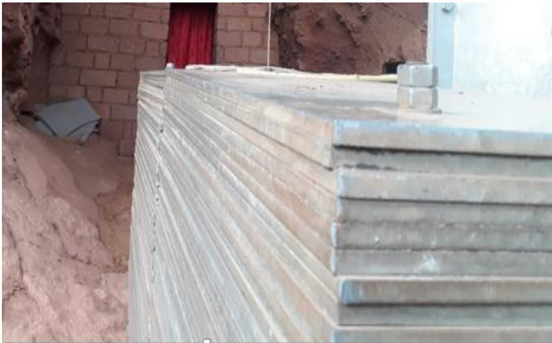
Figure 3.1.1-7:-Column-C1 (It's been witnessed that there are no openings encountered on the base plates but Bending of the base plates is encountered and witnessed).
