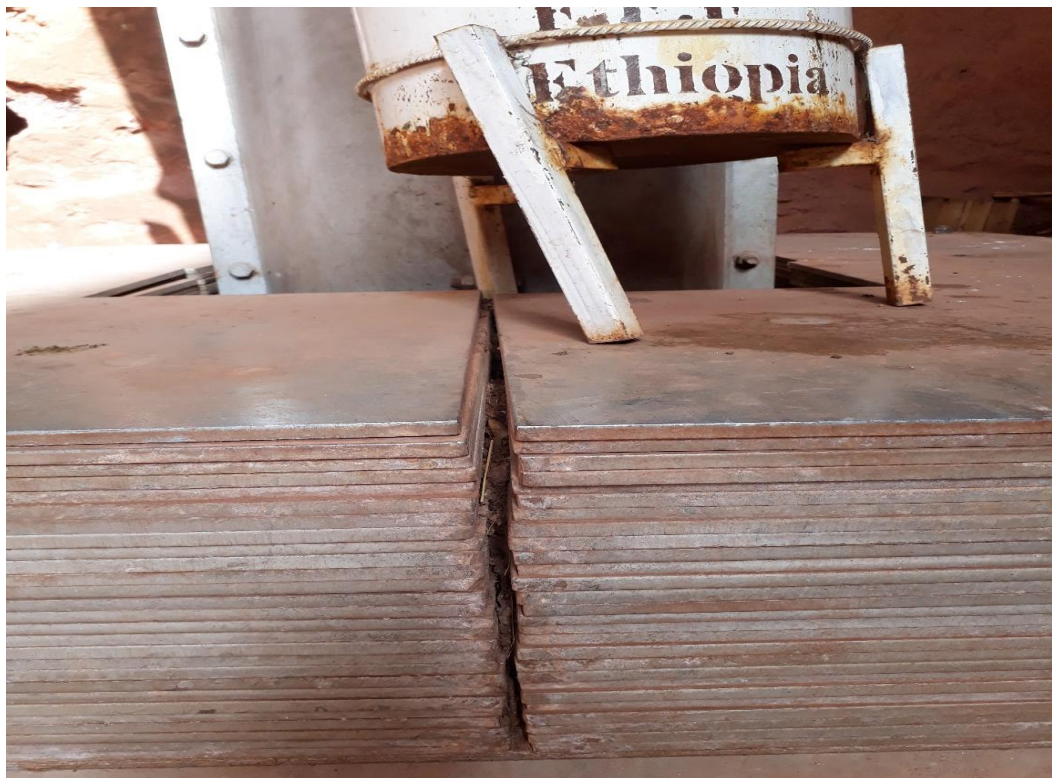
Figure 3.1.1-10:- Column-D2 (It's been witnessed that different width of openings occurred on the base plates in four direction) (photo by Naol G.).
