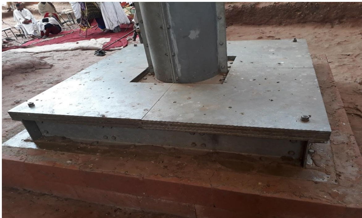
Figure 3.1.1-2 Column-A1 and A3 (it's been witnessed that there are no openings encountered on the base plates)
