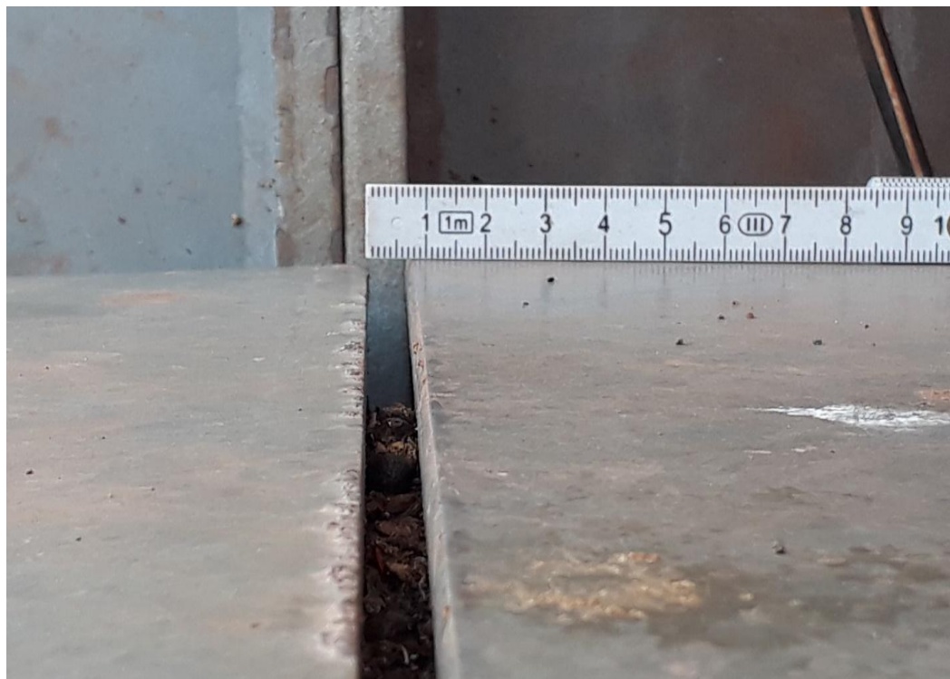
Figure 3.1.1-8:-Column-C2 (It's been witnessed that a slight openings and Bending of the base plates encountered on the base plates in four direction) (photo by Naol G.).
