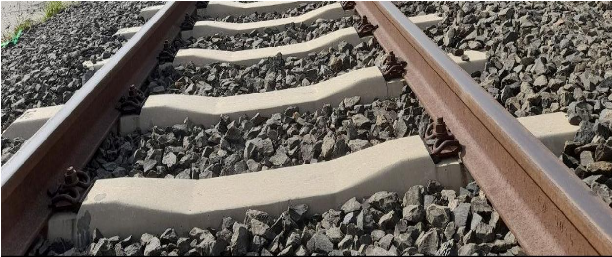
Figure 3.3: Concrete sleeper fixed using UIC 54 rail and SKL rail fasteners at the test site
