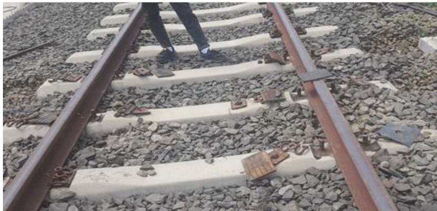
Figure 3.11: Released fastener and rail pad from the tested sleeper
