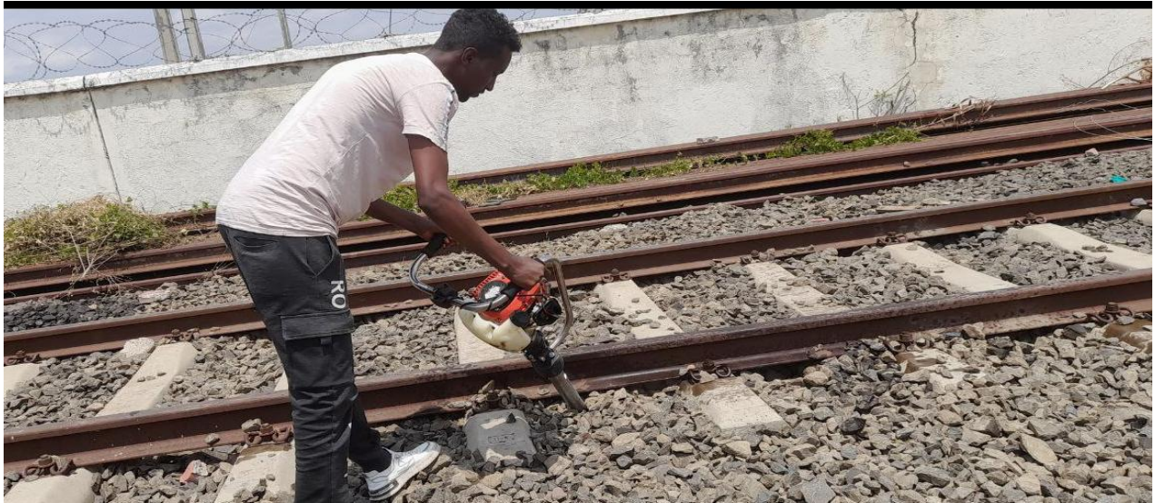
Figure 3.21: Standardized the placement of the tested sleeper and surrounding ballast in the correct position
