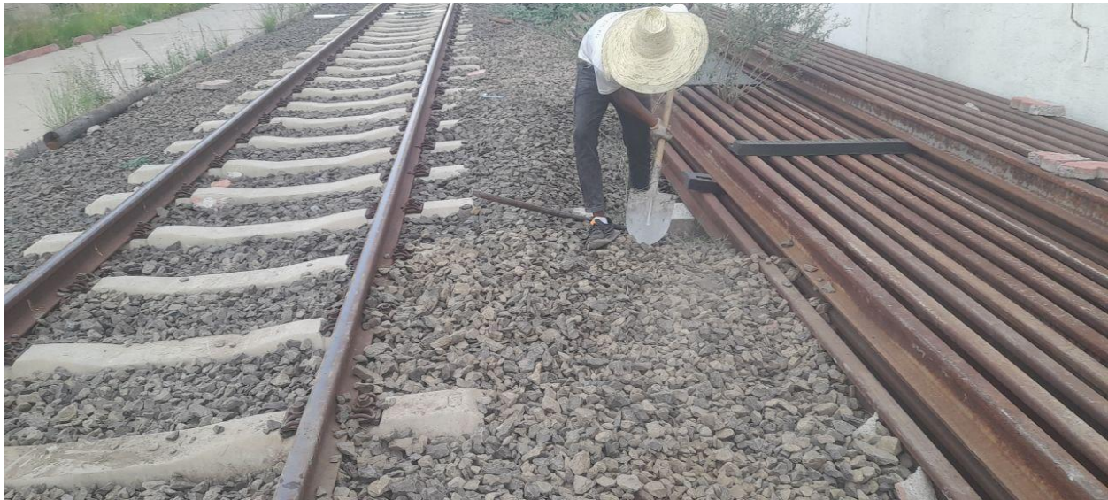
Figure 3.17: Ballast returned, leveled, and sleeper connected to the rail using screw clamp lock fasteners
