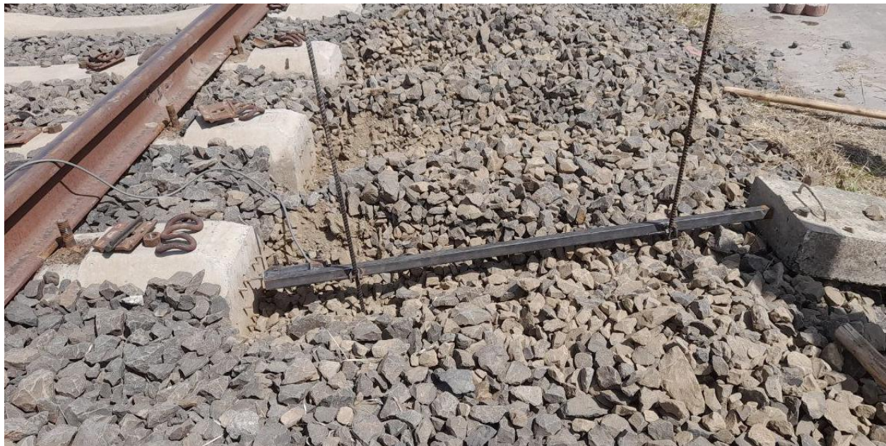
Figure 3.19: Ballast shoulder removed from the tested sleeper and installation of the test instrument
