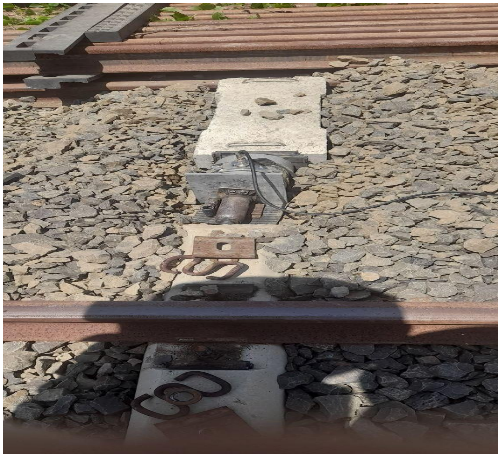
Figure 3.12: Installation of lateral support, load cell, and car crick on one end of the tested sleeper
