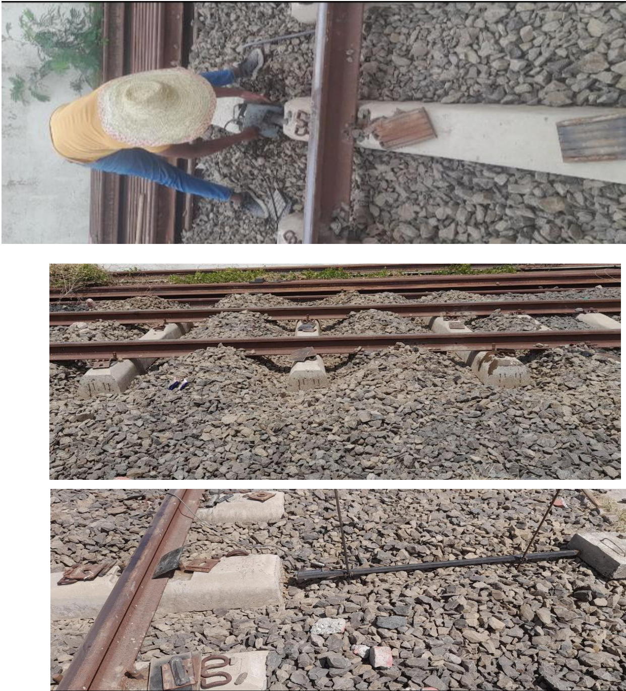
Figure 3.20: Removing the crib and shoulder ballast from the tested sleeper and installation of the test instrument
