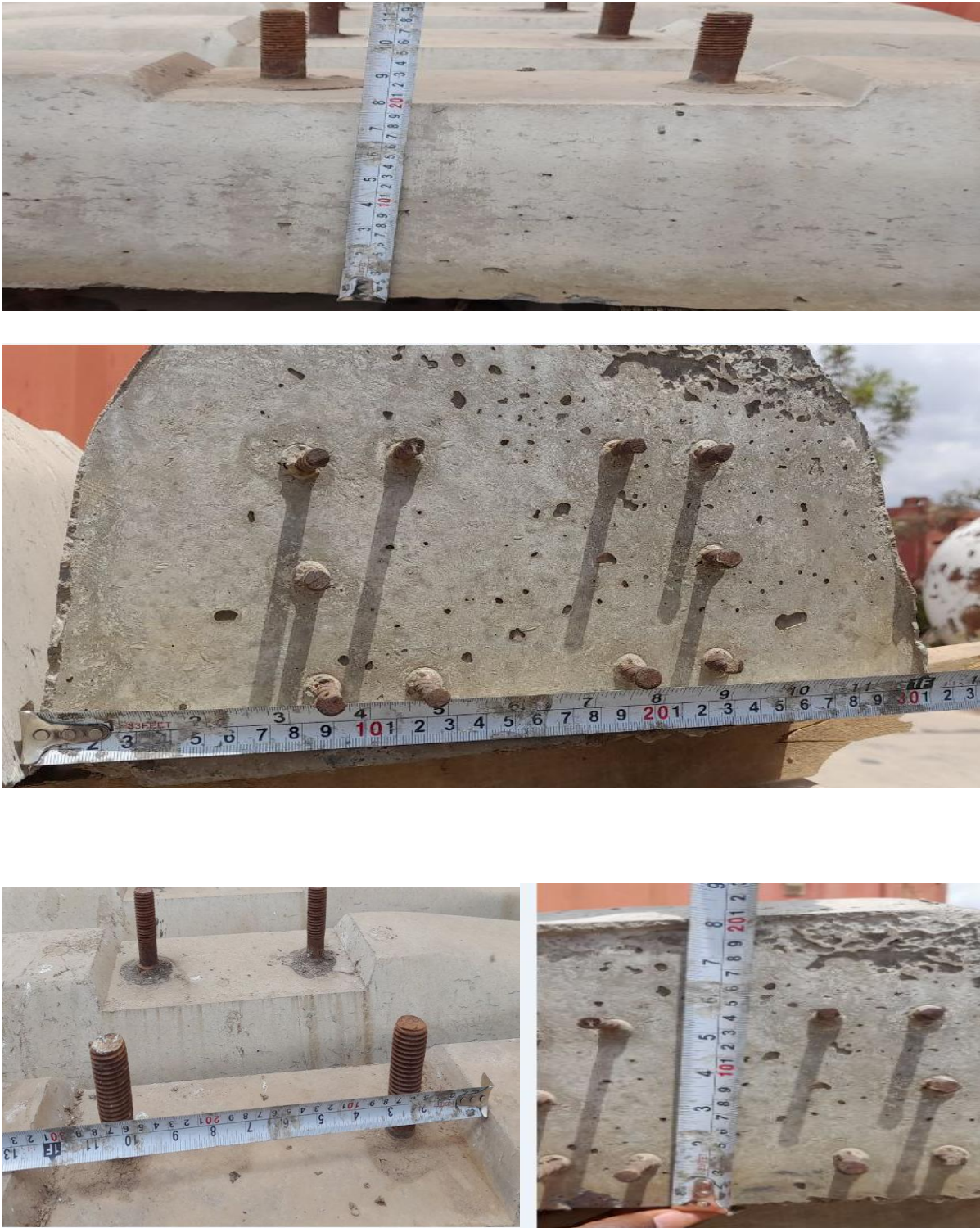
Figure 3.9: Chinese mono-block concrete sleeper (Type-II), detailed dimensional measurements at Indodi Railway Station
