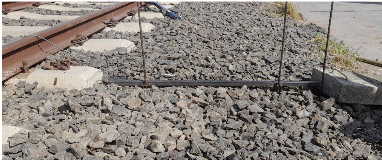
Figure 3.18: Installation of the test instrument and conduct of the test at full section
