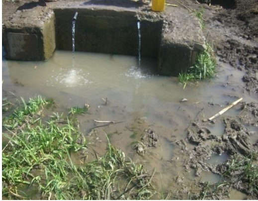
C. Water leaked from hand pipe
