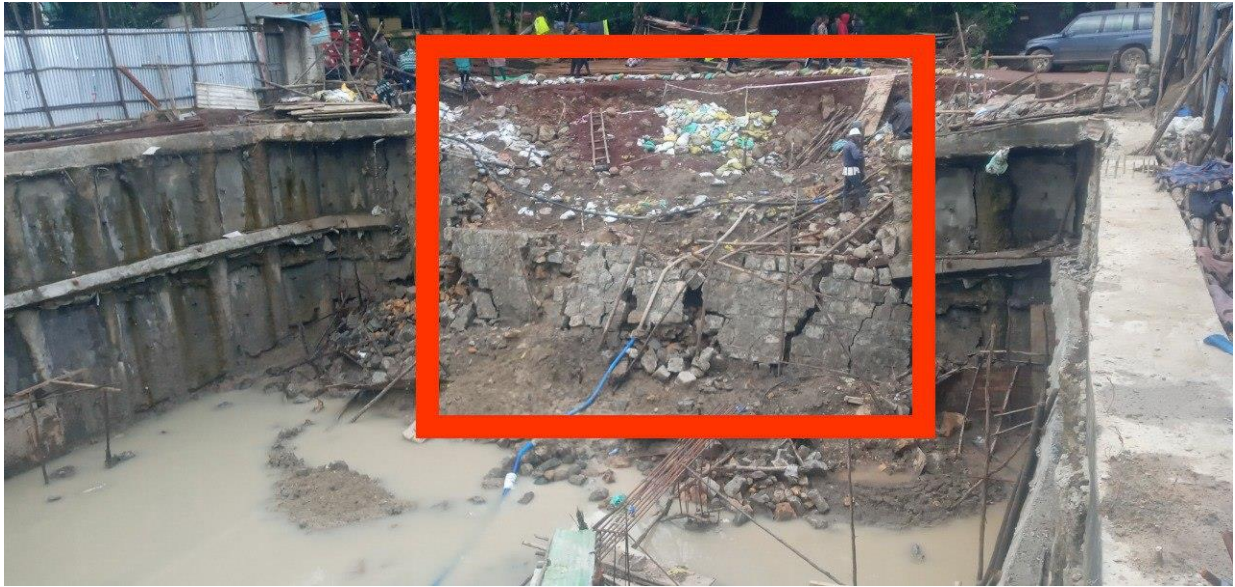
FIGURE 3-2 FAILURE OF MASONRY RETAINING WALL AND EXISTING ROAD IN A. A
