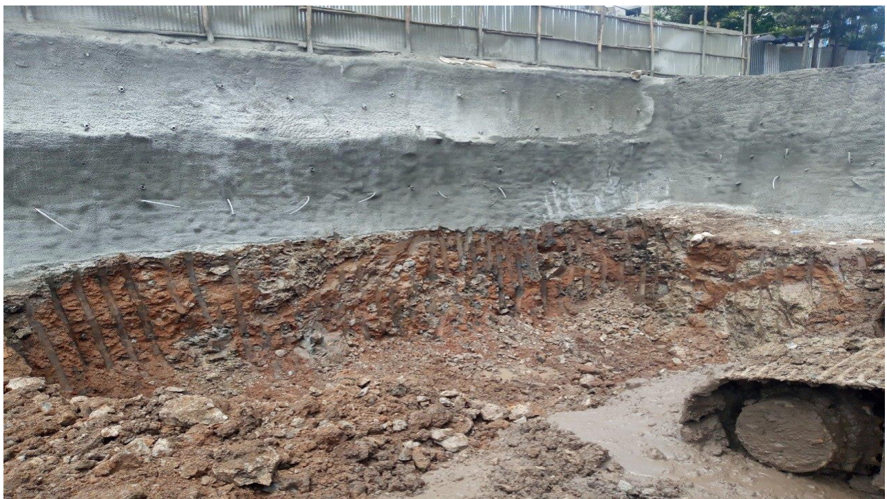
FIGURE 5-24 YEWUB HAGERE PROJECT SOIL NAILING WALL AND ANCHOR BORED PILE WALL VIEW
