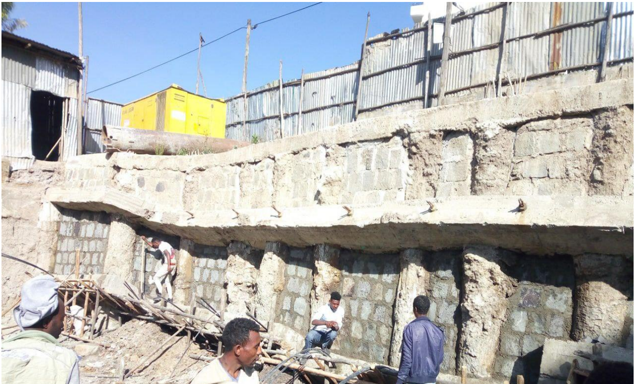
FIGURE 3-20 RCC ANCHOR BEAM WITH MASONRY WALL BETWEEN THE CONTIGUOUS PILES SOIL NAILING WALL
