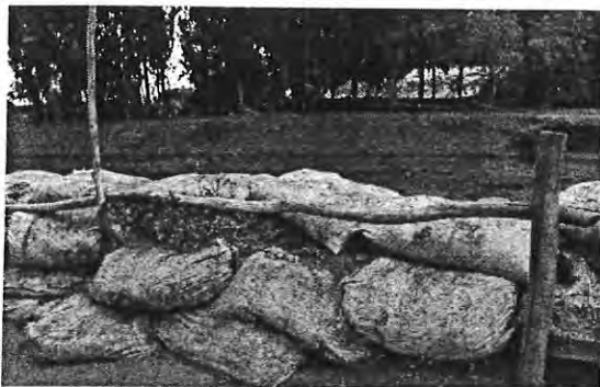
Flood dykes on the river Megech
