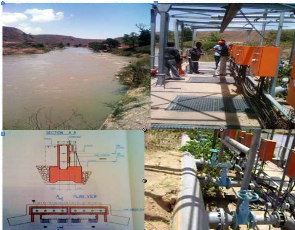
Plate No. 3-1 River Intake and Raw Water Pumping Station
