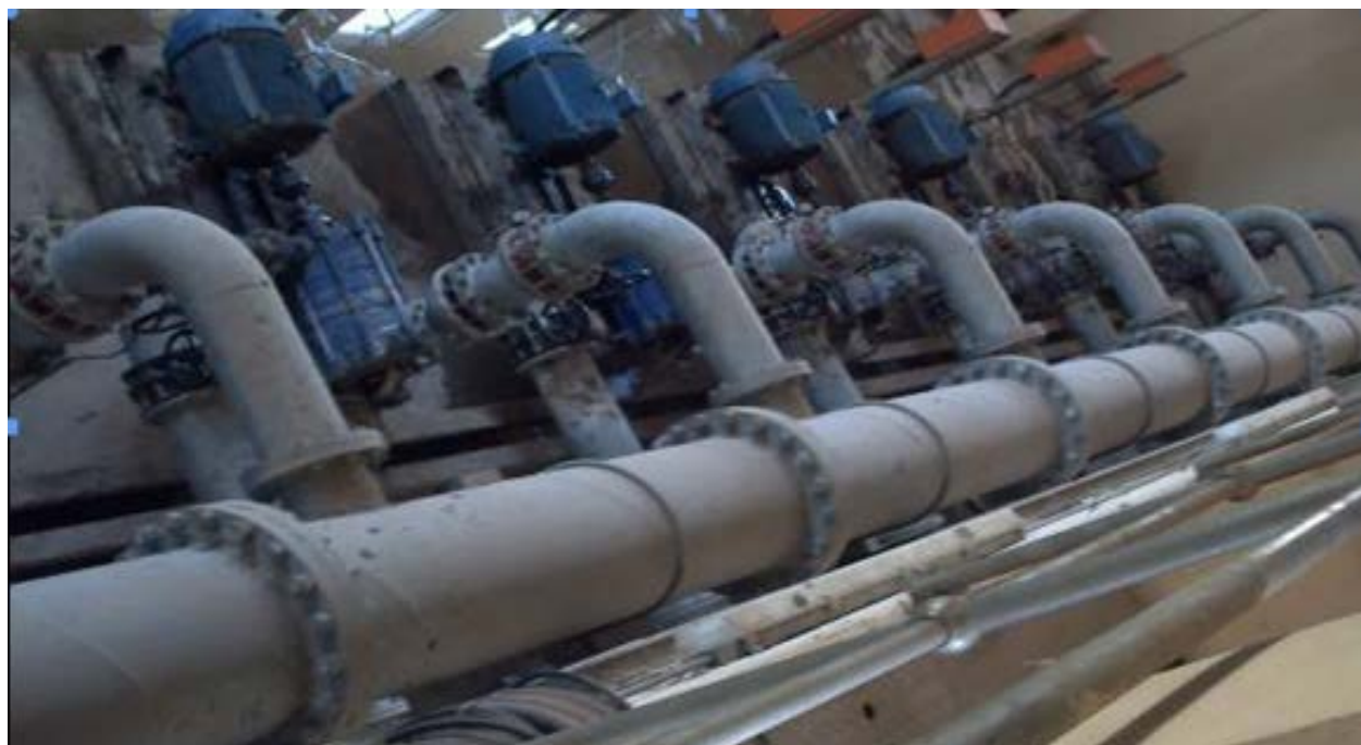
Plate No. 3-4 Partial View of Clear Water Pump Station
