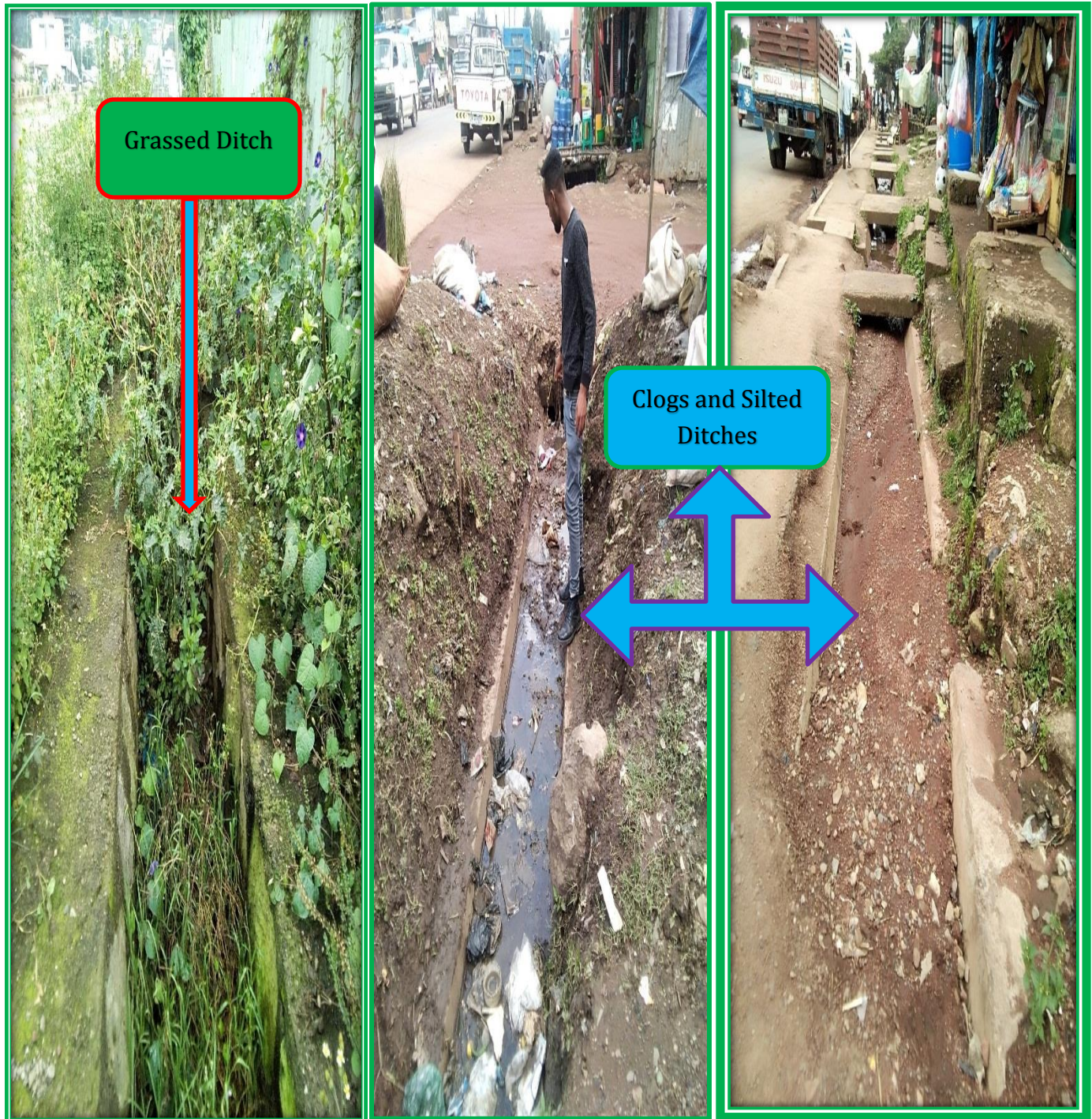
Figure 2-9 : Rectangular type of drainage that is grassed silted and clogs.
