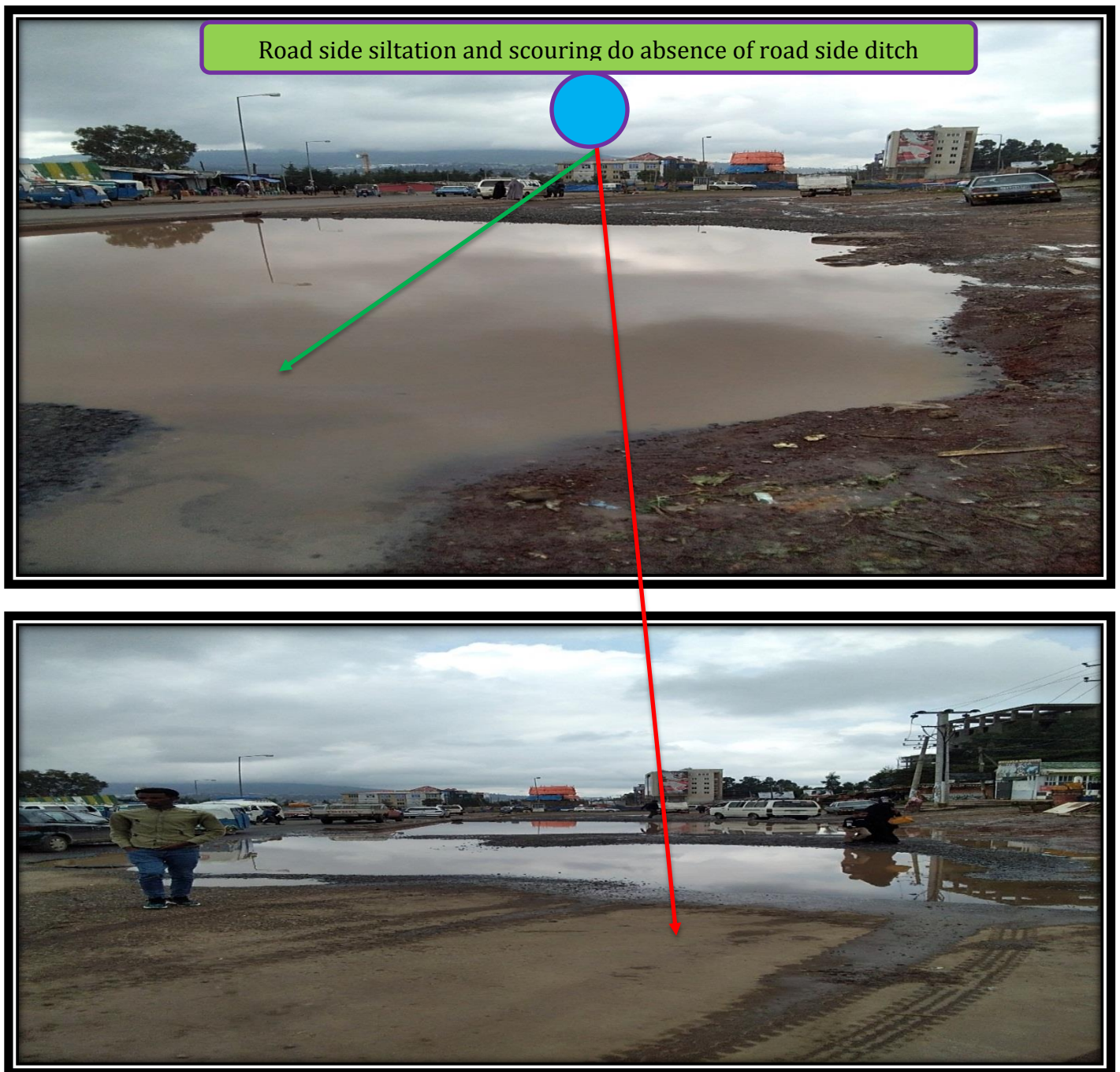
Figure 2-8: Typical Road Failure due to absence of Road side ditch around the Noke in Weleta.
