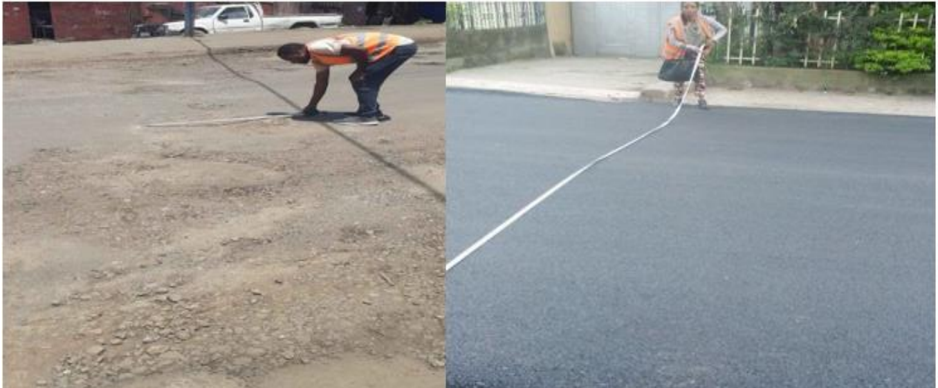
Figure 3-8 Distressed and non-distressed sections of study area
