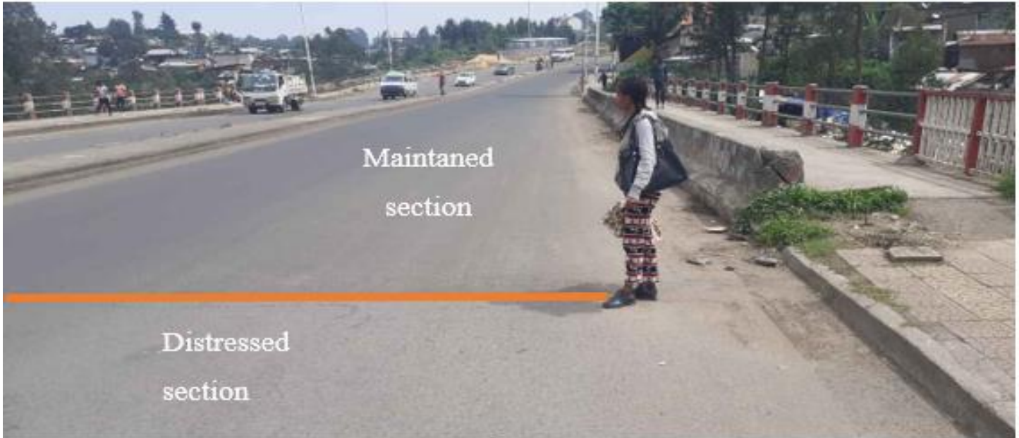
Figure 3-9 the boundary of maintained and distress section
