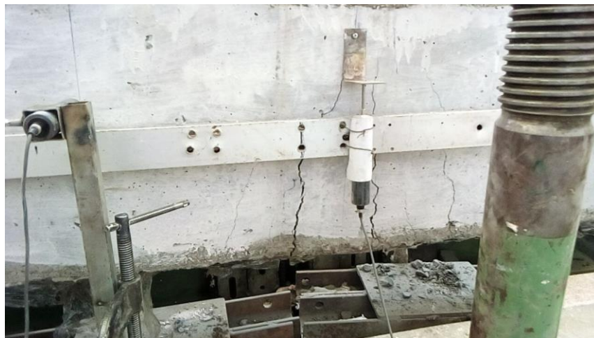
Figure 4-3 bottom Crack (SA-25)
