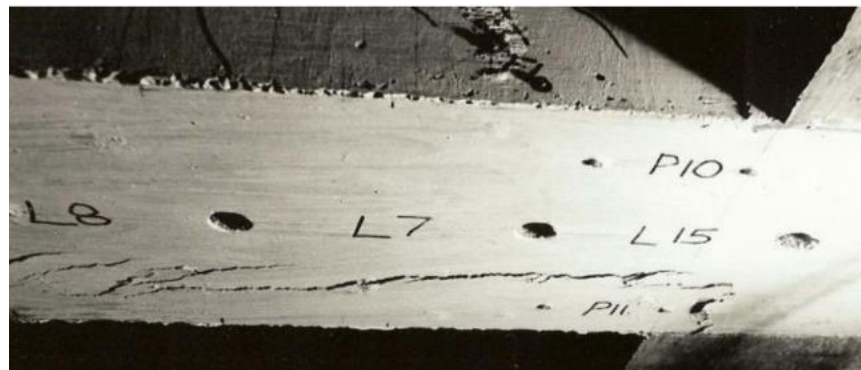
Side Cover Spalling Bottom View
