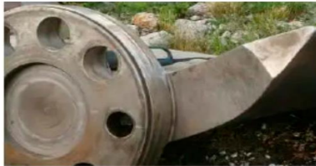
Figure 1.2 the cracked runner blade of a 35.5 MW kaplan turbin in Romania[12]
