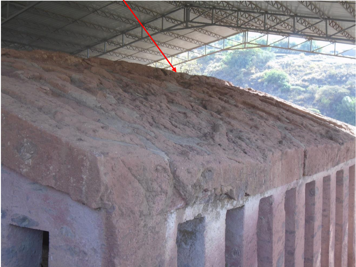
Figure 38: Eroded surface of the roof due to weathering effects. (Source the author)
