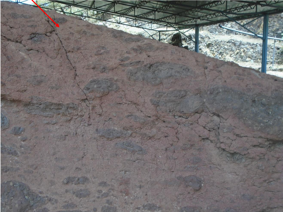
Figure 37. Large cracks on the roof parts of the church. (Source the Author)
