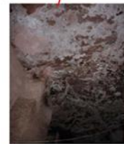
Damages due to water infiltration
