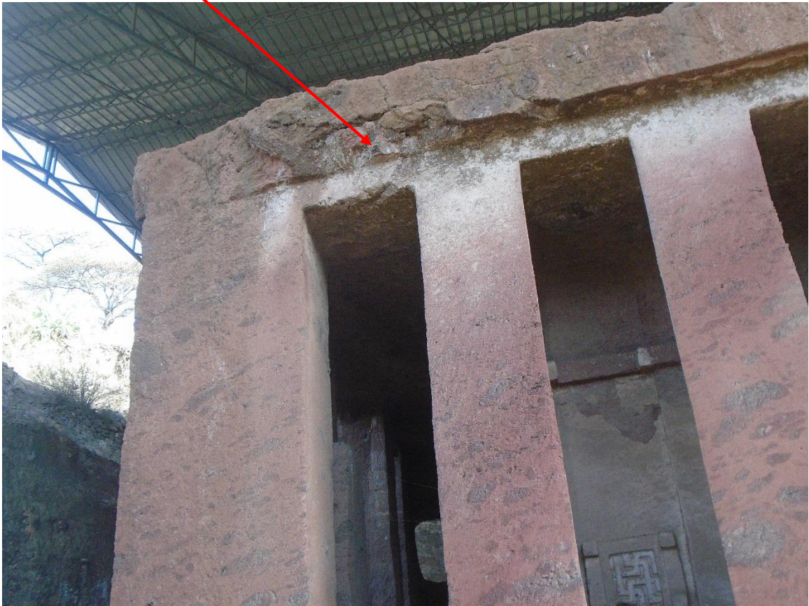
Figure16, Damaged part of the south faced of the church (source the author.)
