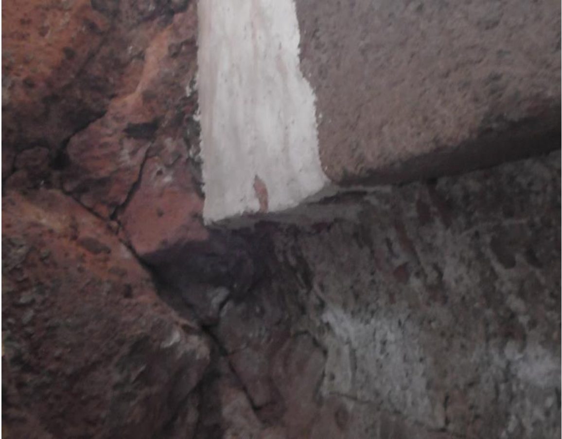
Figure 11, Crack at its roof part of the church, (source the author)
