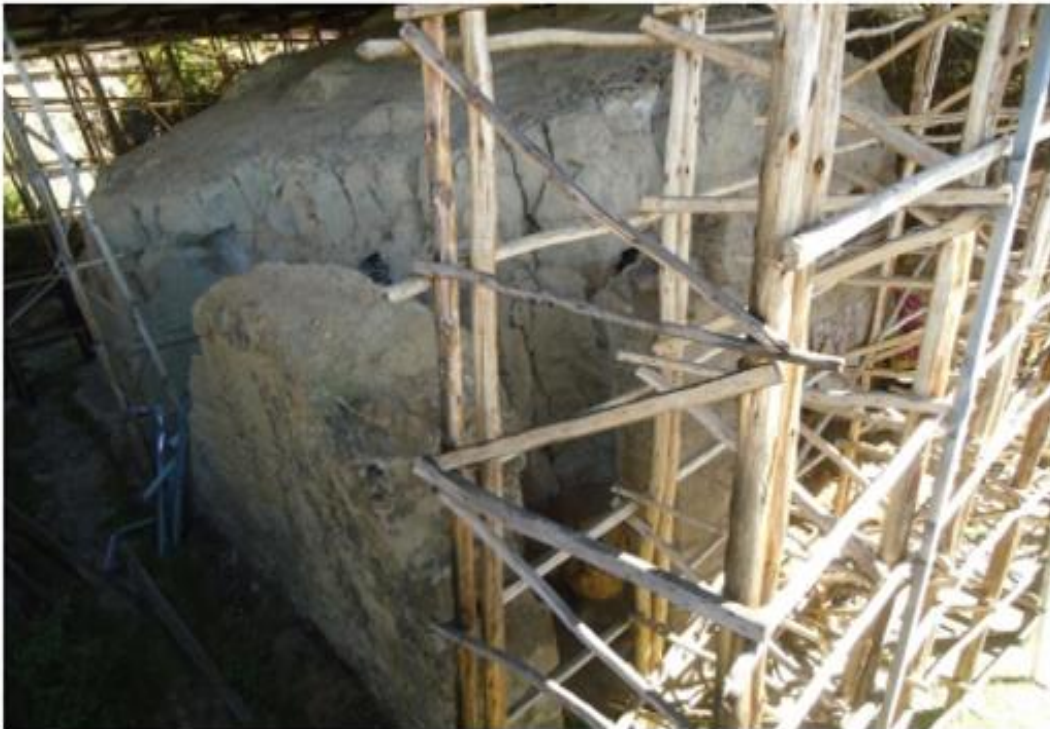
Fig.3. Partial collapse of the church of kenkenit Mikael due to big tree grow on its roof. (Source Lasta culture and tourism office)
