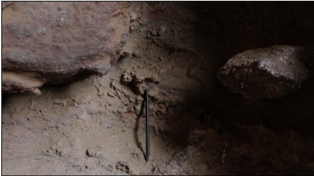
Figure 9: Eroded Part of the church due To the Weathering Process (source the author)
