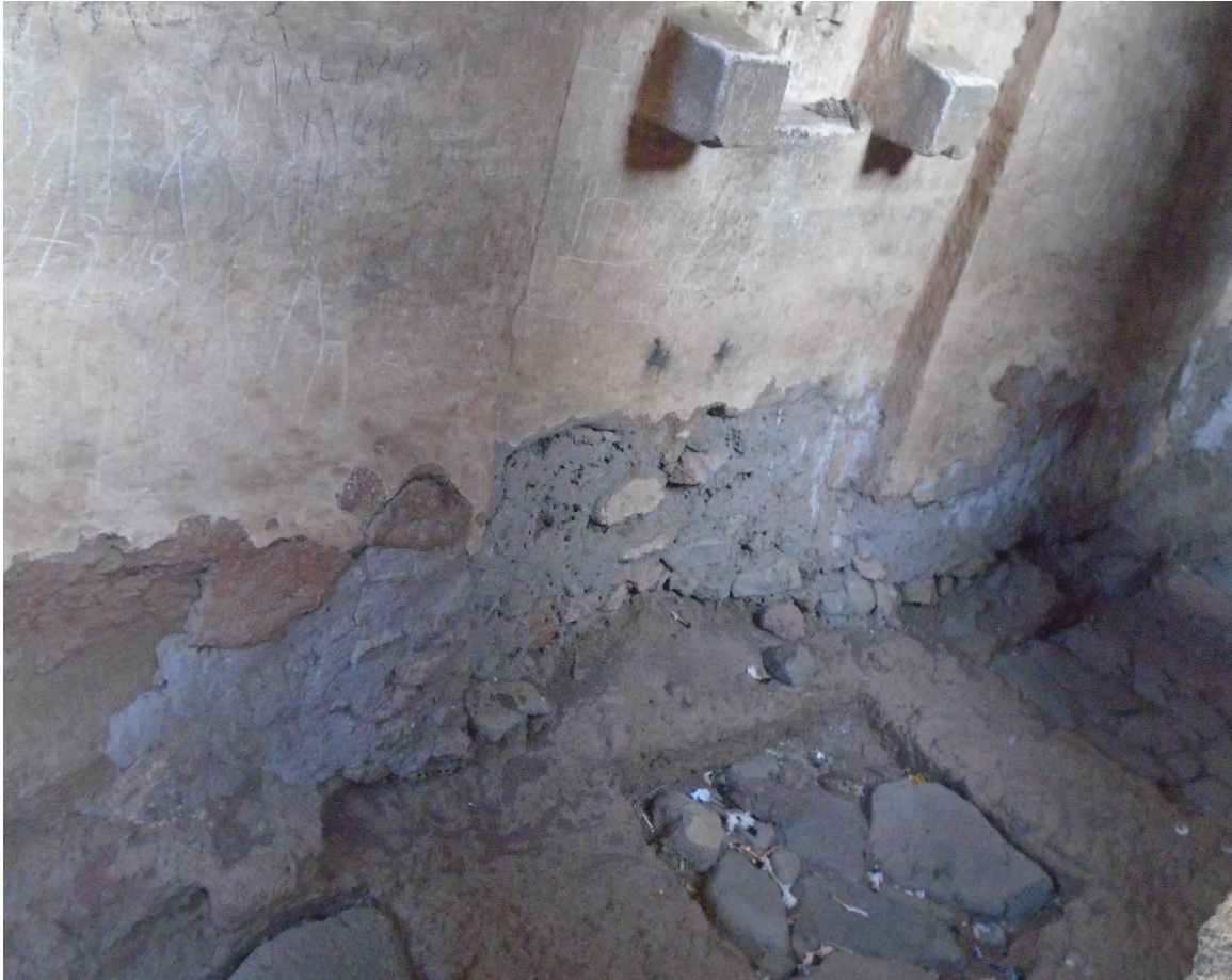
Figure14, Improper Conservation Work at the wall of the Church. (Source the author.)
