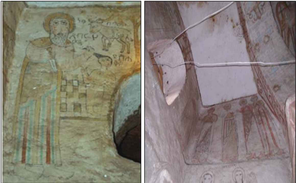
Figure 13: Damage of Wall Painting in the Church (Source the author.)
