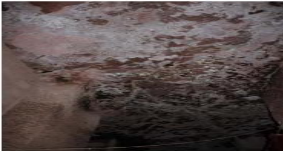
Fig 2: The effect of salt in the church of Arbatu Ensesa at its roof. (Source Lasta woreda Culture and Tourism Office.)
