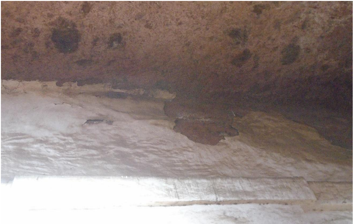
Figure, 12. The plaster are peeled off in many parts inside the church (Source the author)
