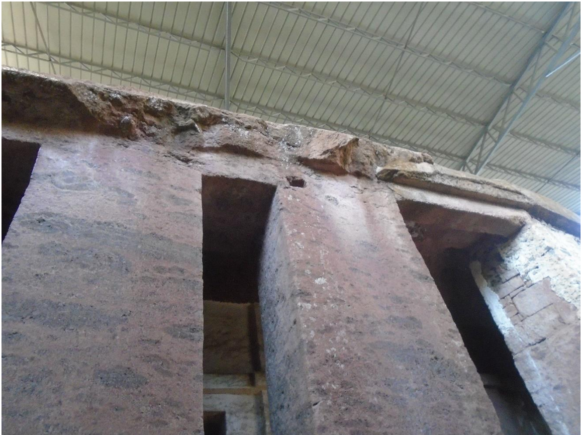
Figure 17, Damage of the rock at its northern faced of the church (source the author)
