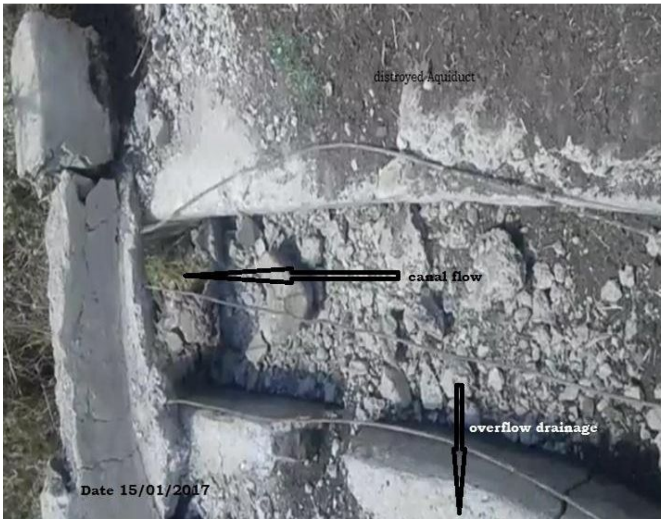
Figure B-4 Veiw of demolished aqueduct in nonfunctional Part of Jemjem SSIP seen during the study
