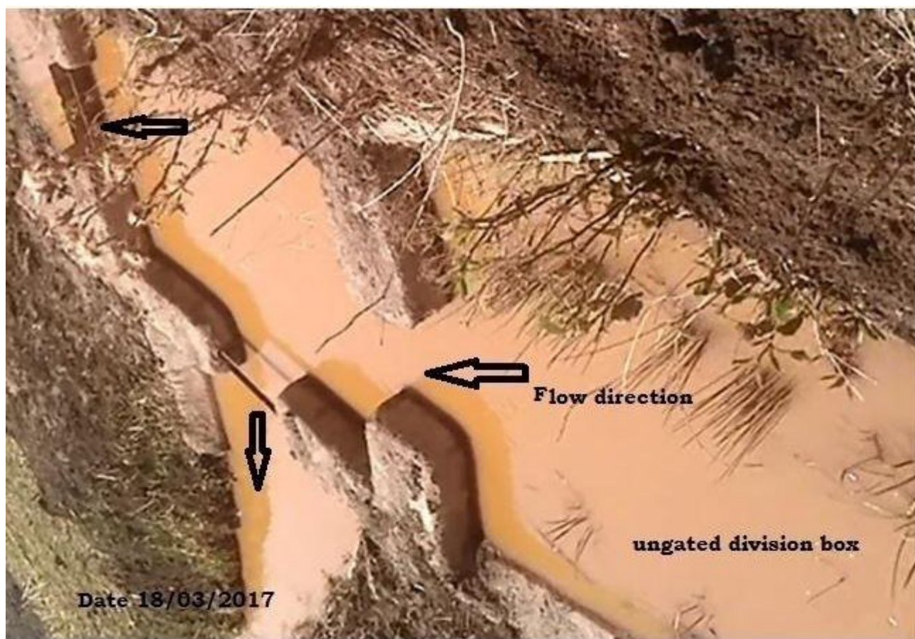
Figure B-1 Division box without gate or uncontrolled water (Jemjem SSIP)
