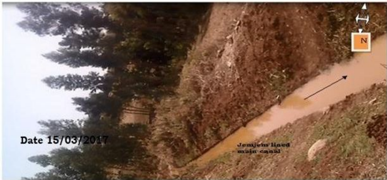
Figure 4.2 Full canal flows as silt deposited in lined part of the MC
