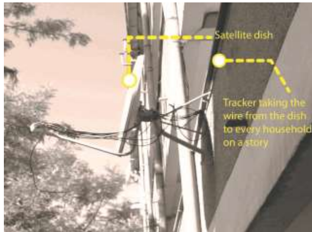
Figure 11: Satellite Dish used in common Groups of 6 to 12 households at Enderase Condominium use one satellite dish in common Source: Own Picture
