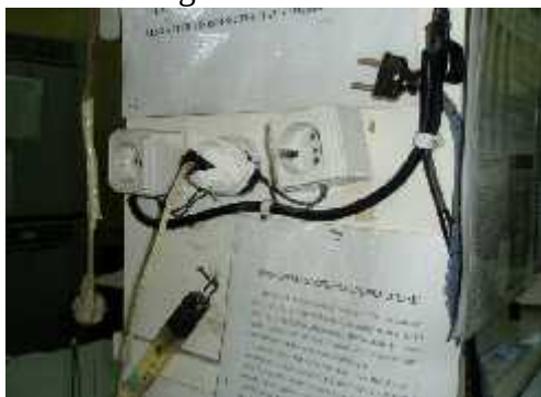
D: Casework wires: no utility core
