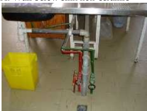
B: Plumbing system
