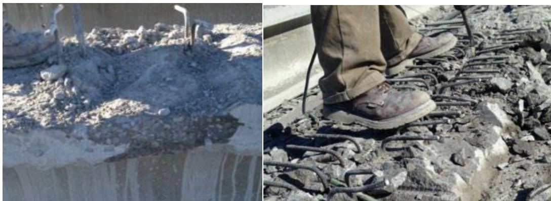
Figure 2. 8 Unintended Construction-Related Damage
