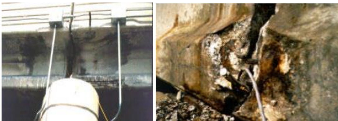
Figure 2. 9 Corrosion and Deterioration of Prestressed Girders
