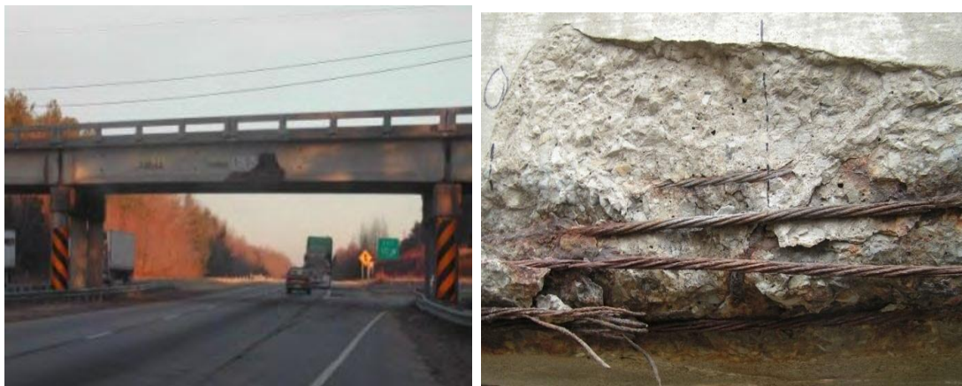
Figure 2. 7 Accidental Impact Damage Due to Over-Height Vehicles
