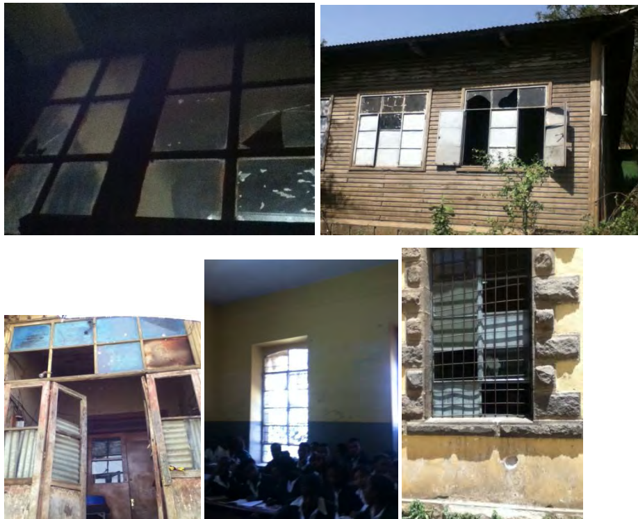
Figure 17: Old Historic Buildings with Broken Windows and Doors in need of Maintenance
