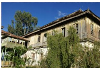
Masonry wall at ground level and wooden post at the upper level at block A
