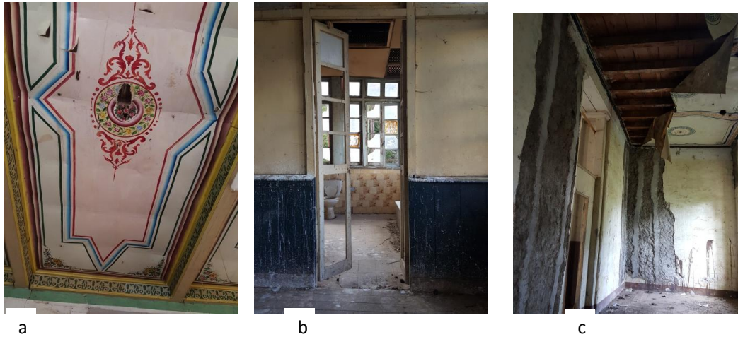
Figure 5.4 – ceiling cover damage
