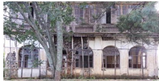
Masonry wall at ground level and wooden post at the upper level at block A
