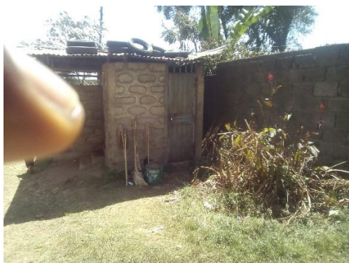
Poor Toilet Service
