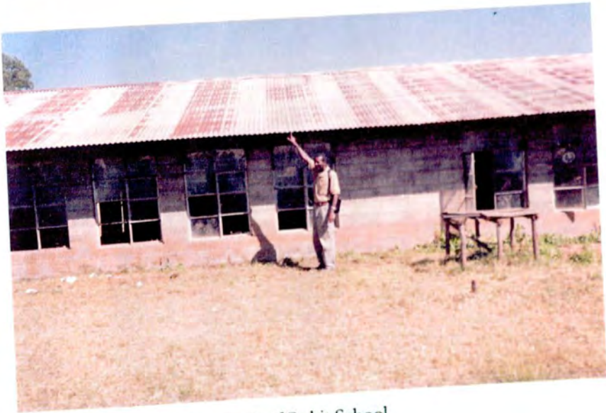
Photo 5.1 Silted up compound of Robit School
