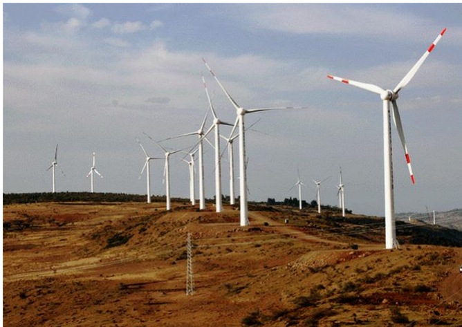
(a) Horizontal Axis wind turbine in Adama I wind-farm in Ethiopia [9]
