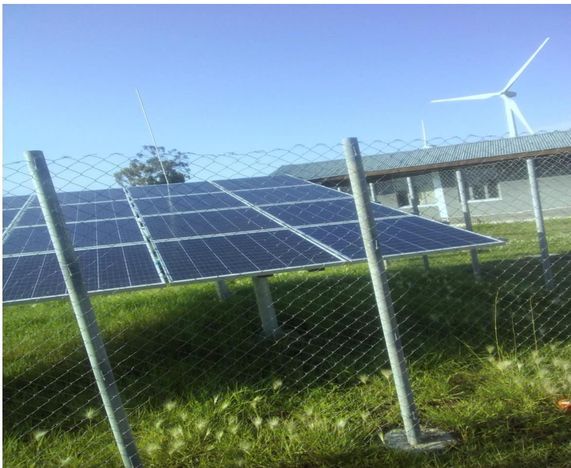
Fig.25.Solar panel 4050 watt that used as source of power for MukoyeHaro health station
