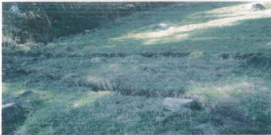
Figure 4.17 Tensional cracks down the road at Shola Wuha locality
