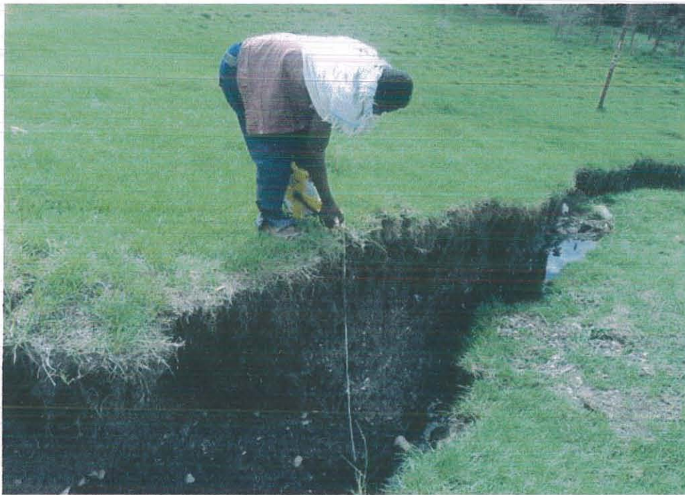
Figure 4.6 Residual clay soils at Shola Wuha locality of the study area showing the deep near vertical fissures.
