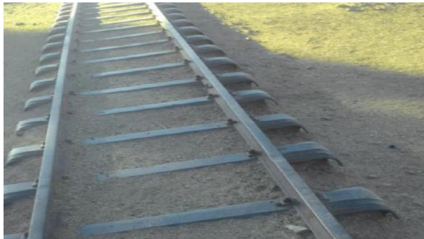
Fig. 3.2. Condition of Ethiopian old railway track
