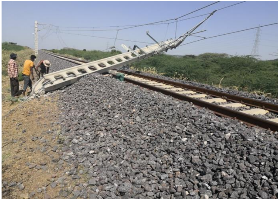
Figure 4.5: Vandalized concrete mast.
