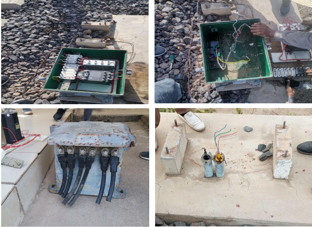
Figure 4.4: Vandalized Track circuit and signaling boxes
